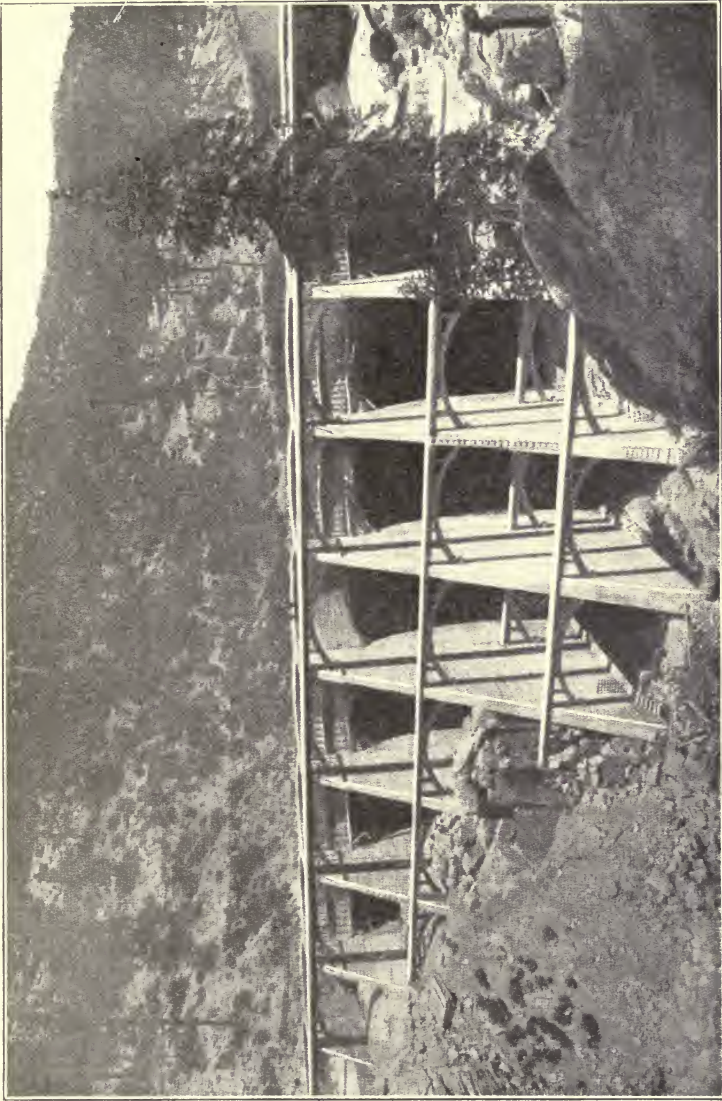
Fig. 78. Back View of Big Bear Valley Dam, Showing Construction of Multiple Arches and Buttresses Courtesy of "Engineering News"
