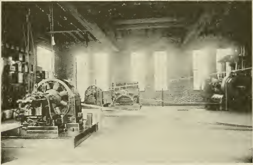
INTERIOR VIEW ELECTRIC LIGHT PLANT
