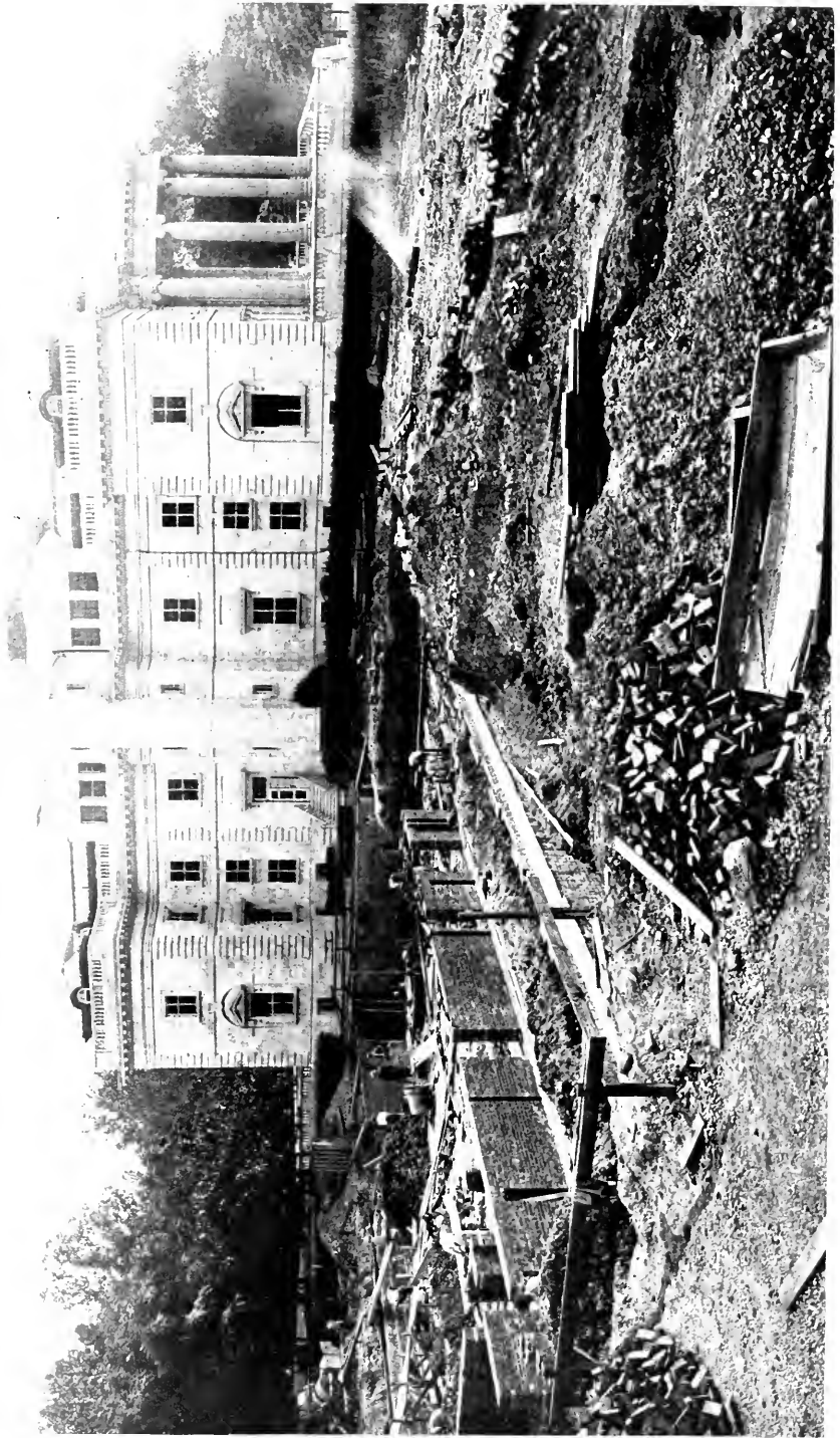
D. A. R. OFFICE BUILDING UNDER CONSTRUCTION GROUND FOR THE NEW STRUCTURE BACK OF MEMORIAL CONTINENTAL HALL WAS BROKEN IN JUNE. IT IS PLANNED TO LAY THE CORNER STONE AT THE OCTOBER MEETING OF THE NATIONAL BOARD OF MANAGEMENT
