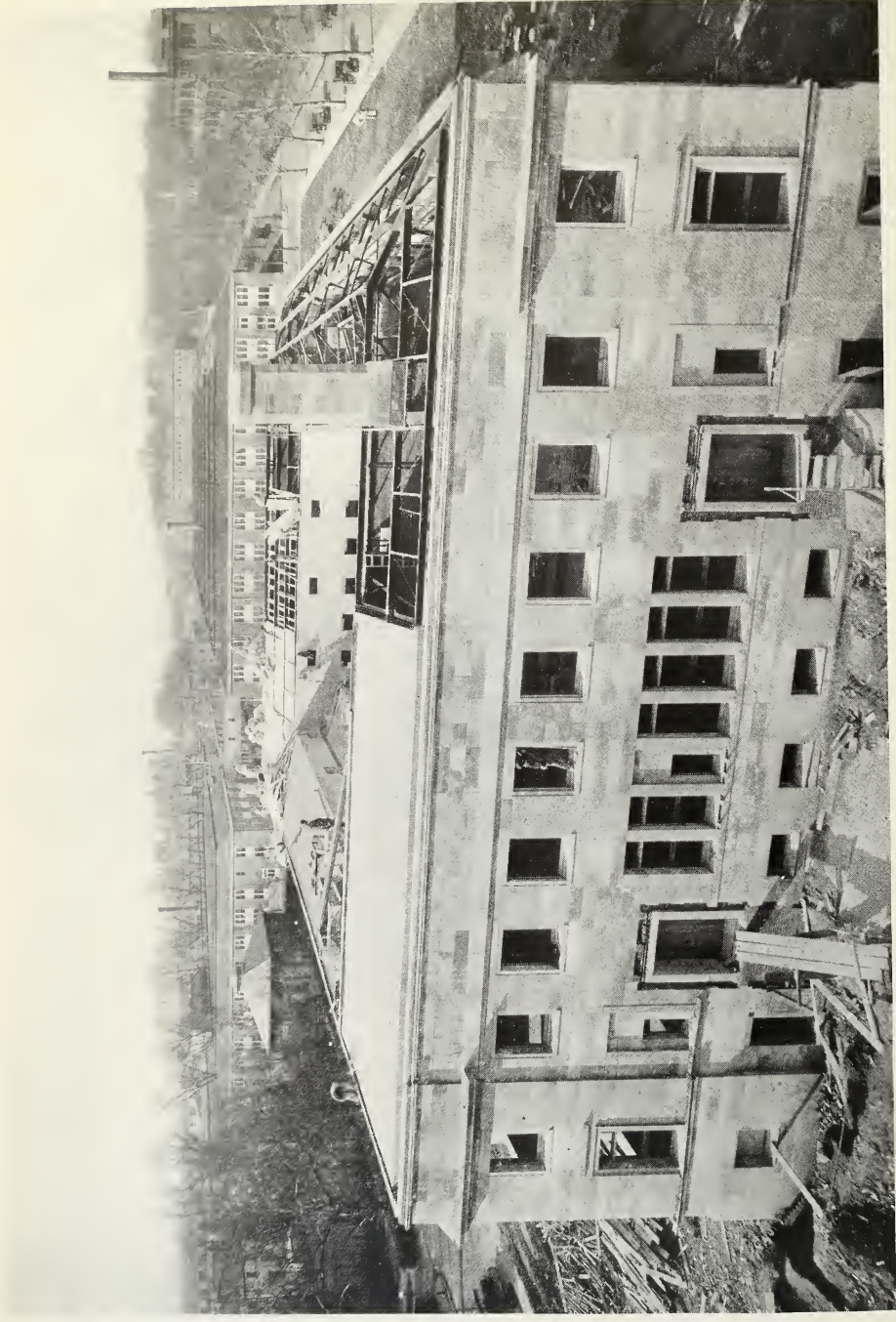
VIEW OF D. A. R. ADMINISTRATION BUILDING LOOKING FROM MEMORIAL CONTINENTAL HALL. THIS VIEW SHOWS THE ROOF CONSTRUCTION
