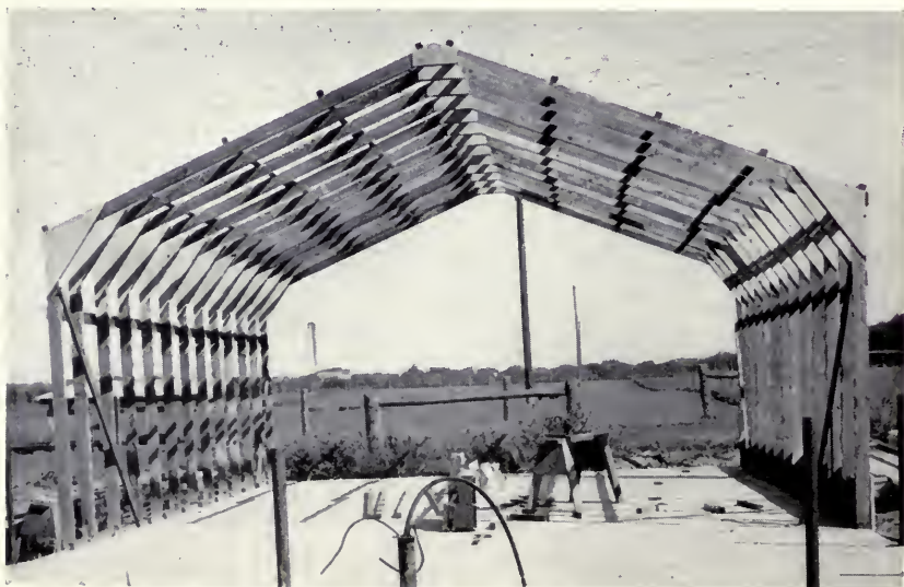
This framework of a small experimental swine shelter shows the type of rigid-frame design being developed. (Fig. 1)
