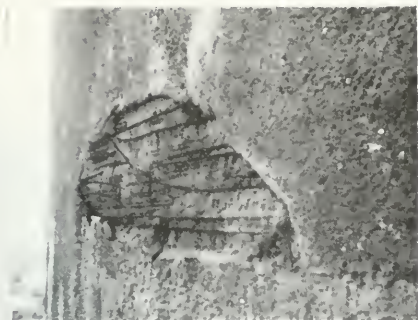
Photo 6-5 Delaminated cover coat exposing broken prestressing wires (AMHERSTBURG)
