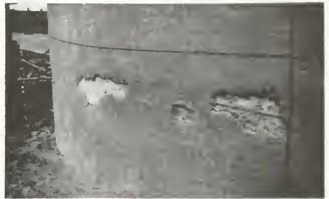
Photo 2-8 External delamination in wire wound post-tensioned tank (WOODVILLE)
