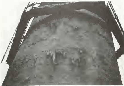
Photo 2-16 Typical horizontal cracks and leachate stains occurring at a prestressed standpipe (WOODVILLE)
