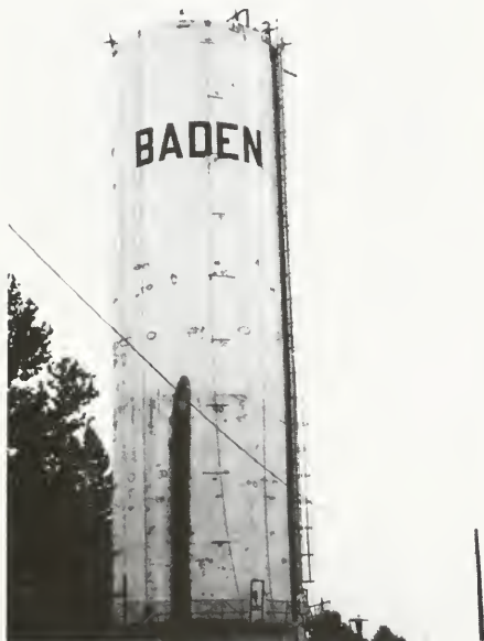
Photo 5-9 Standpipe prior to repair (BADEN)
