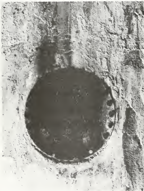
Photo 6-11 Corroded steel manway cover and bolts. (WATFORD)
