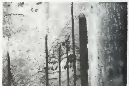
Photo 2-12 Damage caused by water seepage at water-stop (VAL CARON)
