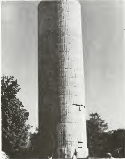
Photo 1-2 Tank implosion. (SOUTHAMPTON)
