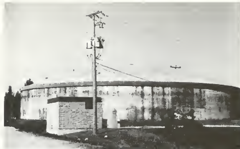
Photo 5-29 Reservoir before repair (PRESTON)
