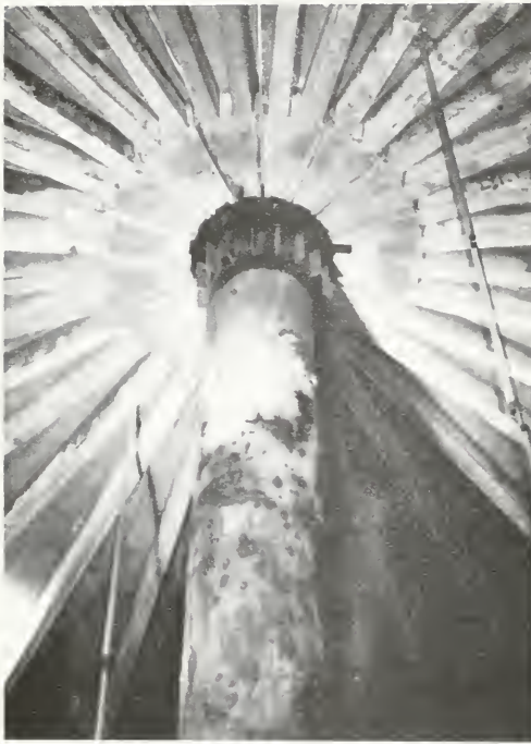
Photo 6-7 Corroded access tube (PRESCOTT)
