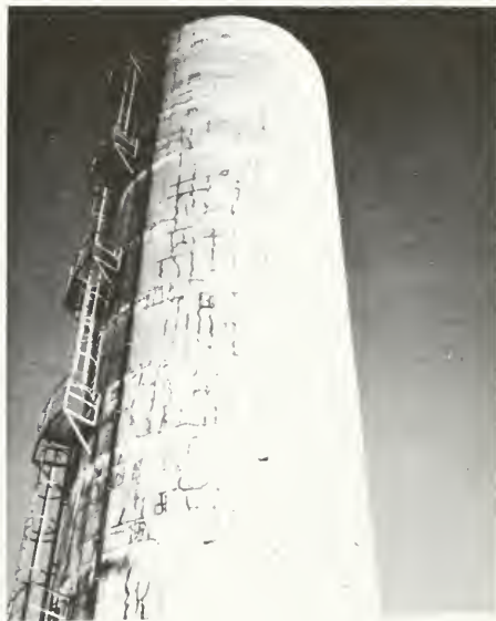
Photo 2-18 Deterioration of reinforced concrete standpipe (ALVINSTON)
