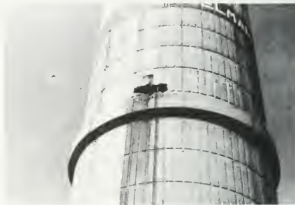
Photo 5-27 Delaminated exterior at source of leak after removal of fractured concrete. (CASSELMAN)
