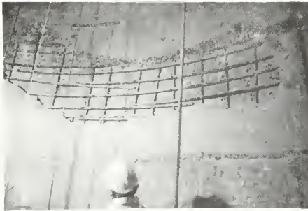
Photo 2-9 Internal delamination (ALVINSTON)
