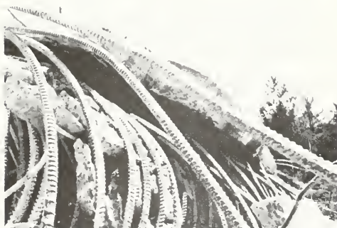
Photo 5-33 Reinforced concrete tank wall after toppling. Note no corrosion of steel and delamination of concrete from steel. (CALLANDER)
