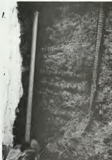
Photo 2-4 Fracture at reinforcing steel (CAMLACHIE)
