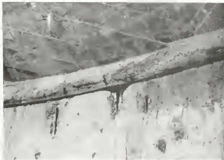
Photo 2-10 Localized spalling (BADEN)
