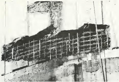
Photo 5-28 Delaminated wall. Inspection revealed ungrouted post-tensioning ducts at this region. (CASSELMAN)
