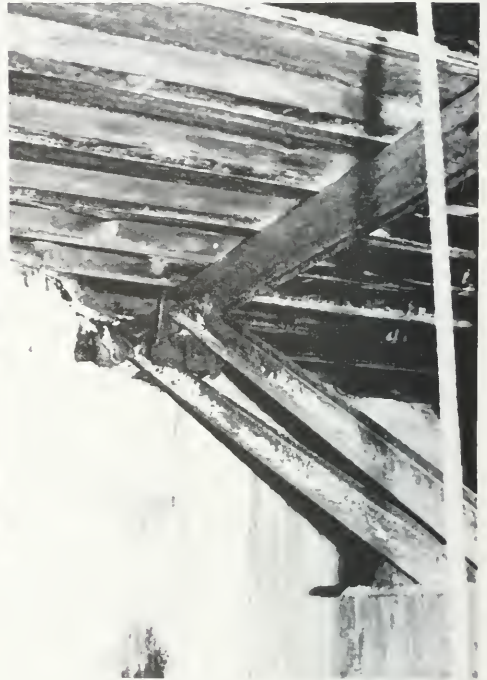
Photo 6-8 Corroded roof truss (HESPELER)
