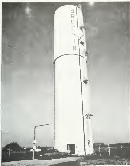
Photo 5-17 Tank after rehabilitation including strengthening by post-tensioning, installation of new steel liner, and insulation and cladding. (BRECHIN)
