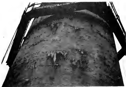
Photo 2-16 Typical horizontal cracks and leachate stains occurring at a prestressed standpipe (WOODVILLE)
