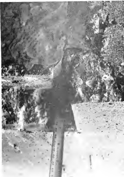
Photo 6-1 Poorly protected post-tensioning anchorage allowing water to enter. (BRIGDEN)
