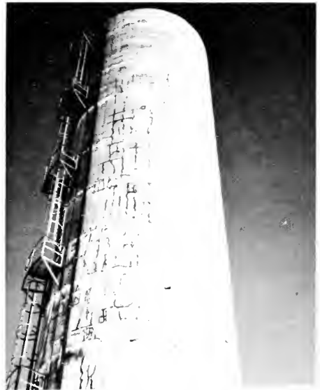
Photo 2-18 Deterioration of reinforced concrete standpipe (ALVINSTON)
