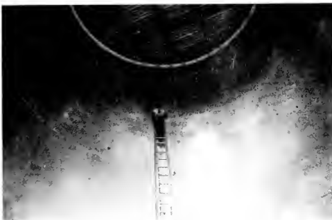
Photo 5-18 Internal maintenance inspection of liner paint system after one year in service (BRECHIN)
