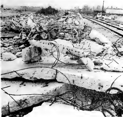
Photo 1-1 Collapsed tank (DUNNVILLE)
