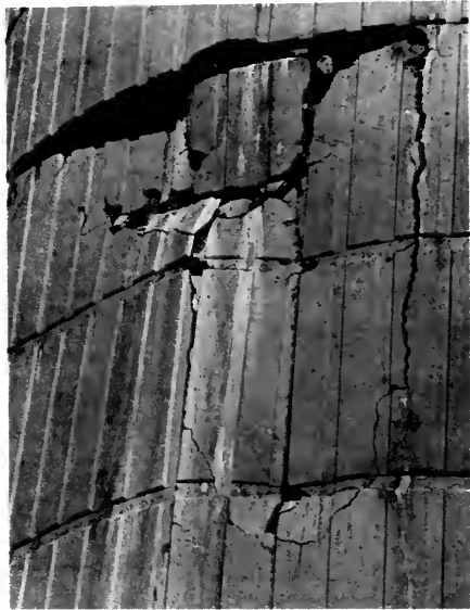
Photo 1-3 Detailed view of imploded section. (SOUTHAMPTON)
