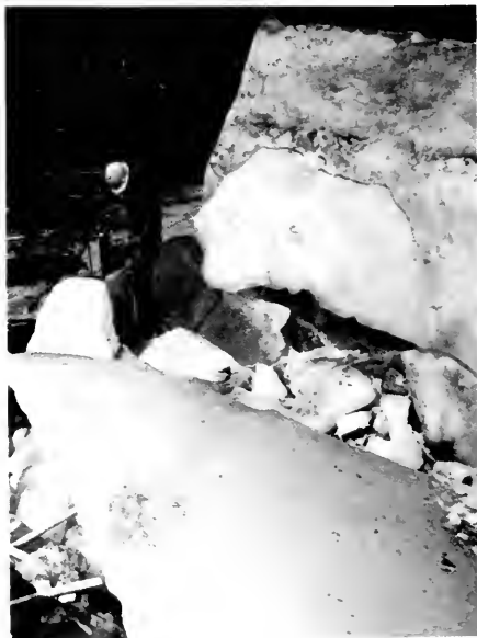
Photo 5-1 Internal wall ice at bottom of tank after demolition in late spring
