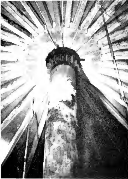
Photo 6-7 Corroded access tube (PRESCOTT)
