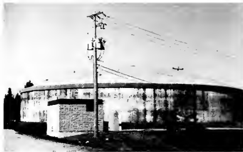
Photo 5-29 Reservoir before repair (PRESTON)
