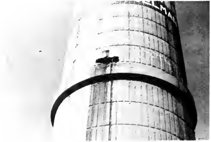
Photo 5-27 Delaminated exterior at source of leak after removal of fractured concrete. (CASSELMAN)
