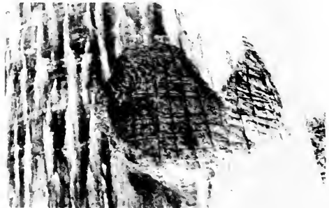
Photo 2-2 External wall delamination (WATFORD)
