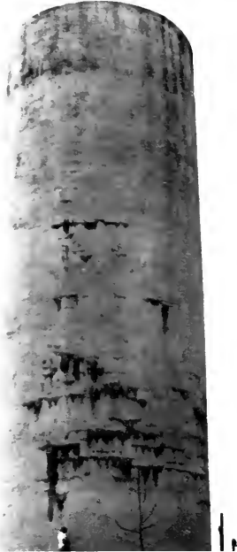
Photo 5-7 Typical horizontal cracking of a G-S type tank. (L'ORIGINAL)
