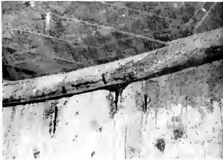
Photo 2-10 Localized spalling (BADEN)
