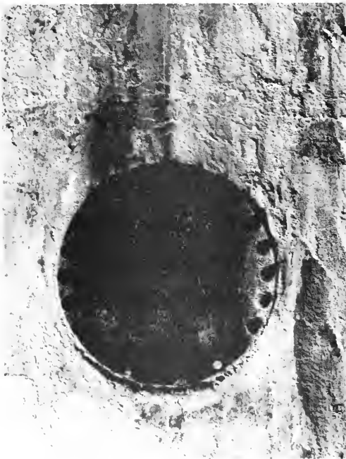
Photo 6-11 Corroded steel manway cover and bolts. (WATFORD)
