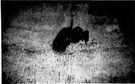
Photo 2-13 Coating deterioration and a jack-rod spall (WOODVILLE)
