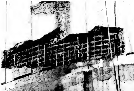
Photo 5-28 Delaminated wall. Inspection revealed ungrouted post-tensioning ducts at this region. (CASSELMAN)
