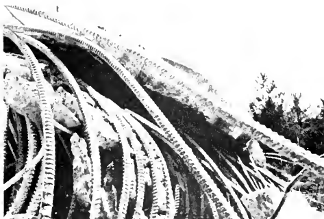
Photo 5-33 Reinforced concrete tank wall after toppling. Note no corrosion of steel and delamination of concrete from steel. (CALLANDER)
