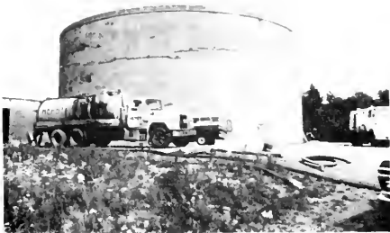
Photo 2-17 Typical cracks and leachate stains occurring at a prestressed ground tank (VAL CARON)
