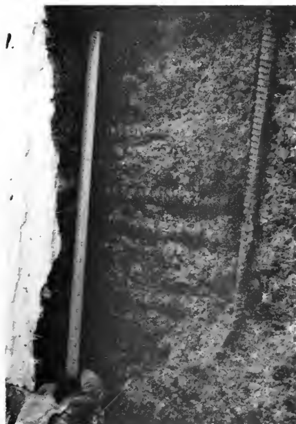
Photo 2-4 Fracture at reinforcing steel (CAMLACHIE)
