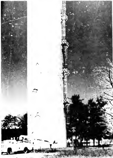
Photo 2-1 Typical deterioration at bottom of reinforced concrete standpipe (WATFORD)
