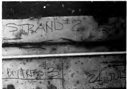
Photo 6-2 Detailed view of strand showing corroded wires. (BRIGDEN)
