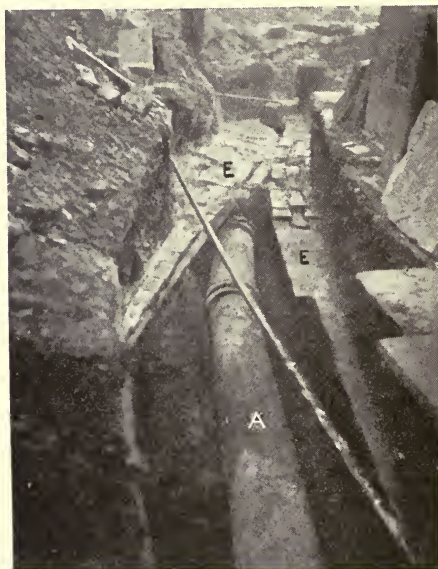
FIG. 132.—Gas Mains Covered over by Electric Cables.
