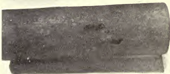
FIG. 685.—Electrolytic Pitting on 3-inch Cast-Iron Main.
