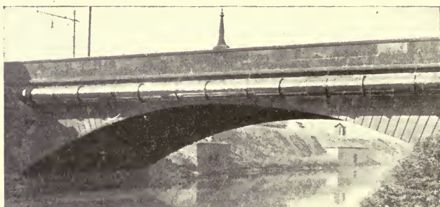
FIG. 53.—Elevation of 36-inch Steel Main over River Aire, at New Wortley, Leeds.
