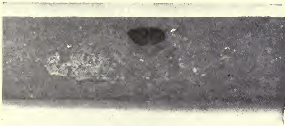
FIG. 670.—1-inch Service Pipe Fused by Tramway Cables at Leeds.
