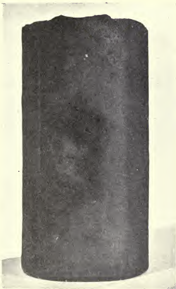
FIG. 684.—Electrolytic Pitting on 4-inch Cast-Iron Main.
