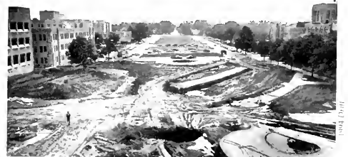
Renovations In attempts to beautify the campus, sidewalks, trash cans as well as benches were installed after the demolishing of the grounds between Jordan and Holcomb.
