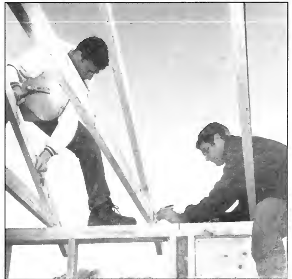
Seniors Andrew Torrella and Paul Babcock nail a beam to the roof of the house.
