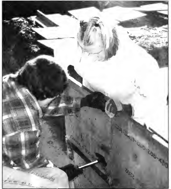
Senior Rachel Mohlman and Junior Sara Lusk set up a board so they can pour concrete.
