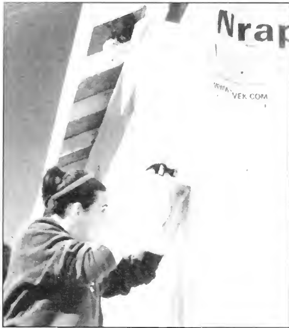
Cathy Giorgio is having fun as she nails a board to the house.
