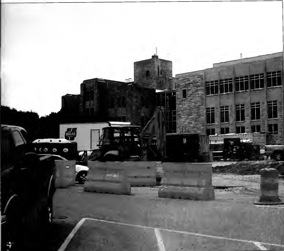
A picture of the Pharmacy building was taken towards the end of construction. Students watched to building go from empty shell to an all new green space.
