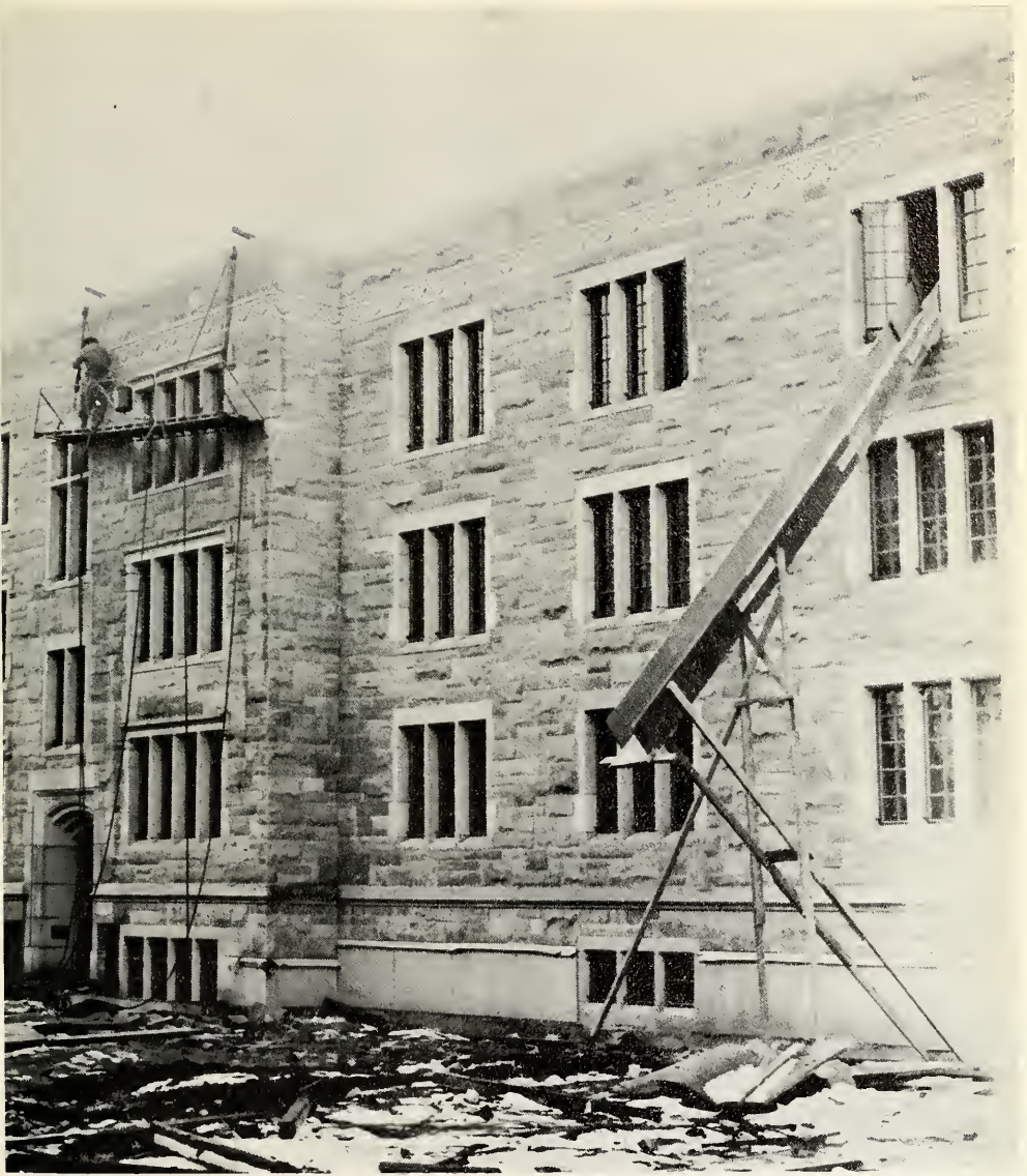
Seen here is one end of the new men's dormitory, built for the university by the Air Force. While the dormitory is primarily for the use of the AFROTC students, living quarters will be available to any Butler man desiring to stay there.
