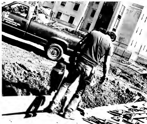
Construction workers set the forms up as they prepare to pour the new curbs to the remodeled mall.
