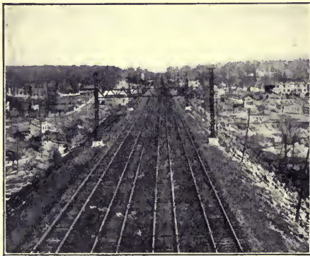
Electrification on the New York, New Haven and Hartford Railroad. Overhead Transmission.
