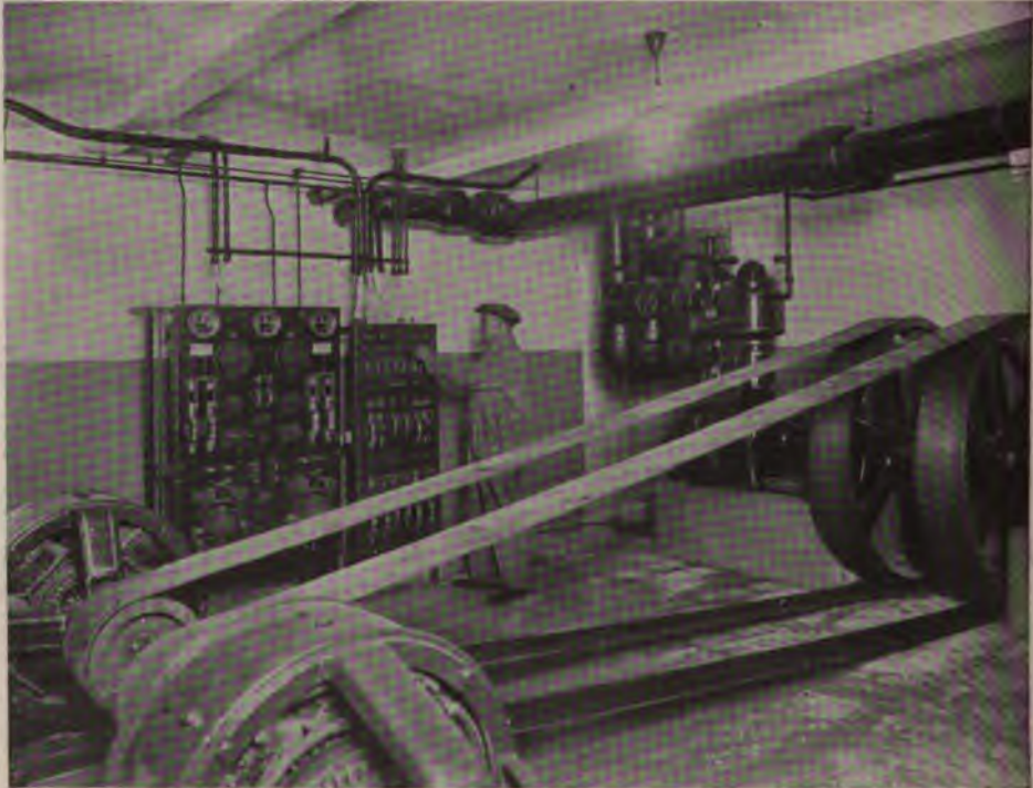
Photograph by The New York Edison Company
