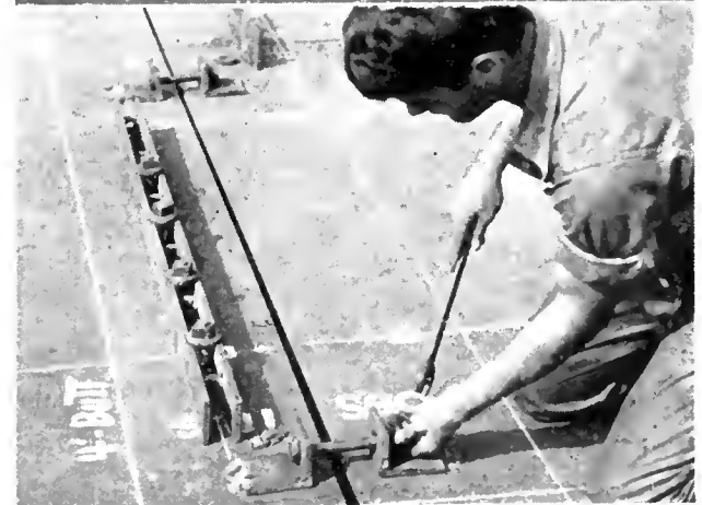
Shipbuilding Skills: (Top to bottom) "Interbottom Sections;" "Side Frames—Sub-assembly of a Web Frame;" Deck Girders;" "Deck Plates—Regulating and Setting."
