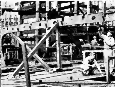
Two scenes at left show fitting and fairing of floors and longitudinals into an innerbottom.
