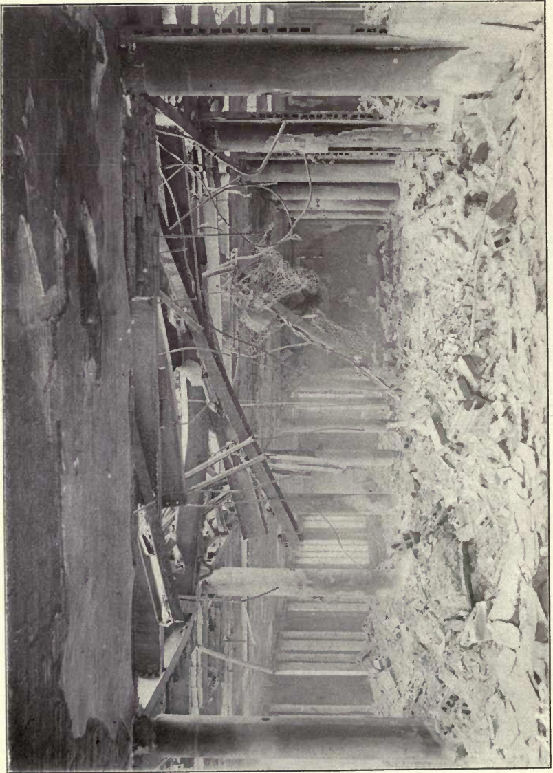
TENTH STORY, Looking North, Showing Condition on Eleventh Floor on Account of Collapse of Columns 33 and 34. Cylinder Press Hanging in Eleventh Floor Shown in Rear.
