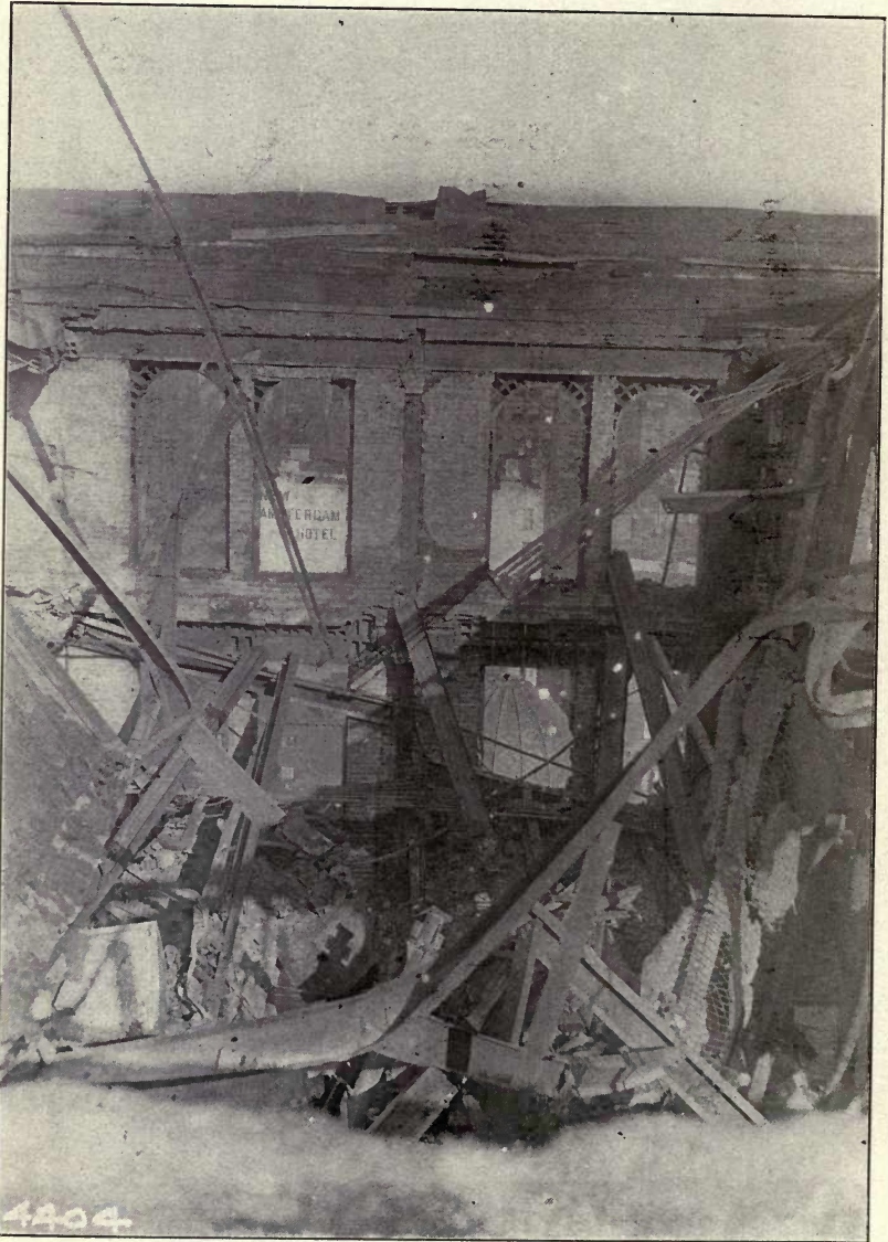
4404 TWELFTH STORY, Looking North, Showing Collapsed Portion of Roof, Vicinity of Columns 33 and 34, Damaged Cornice, Exposed Wall Columns, etc.
