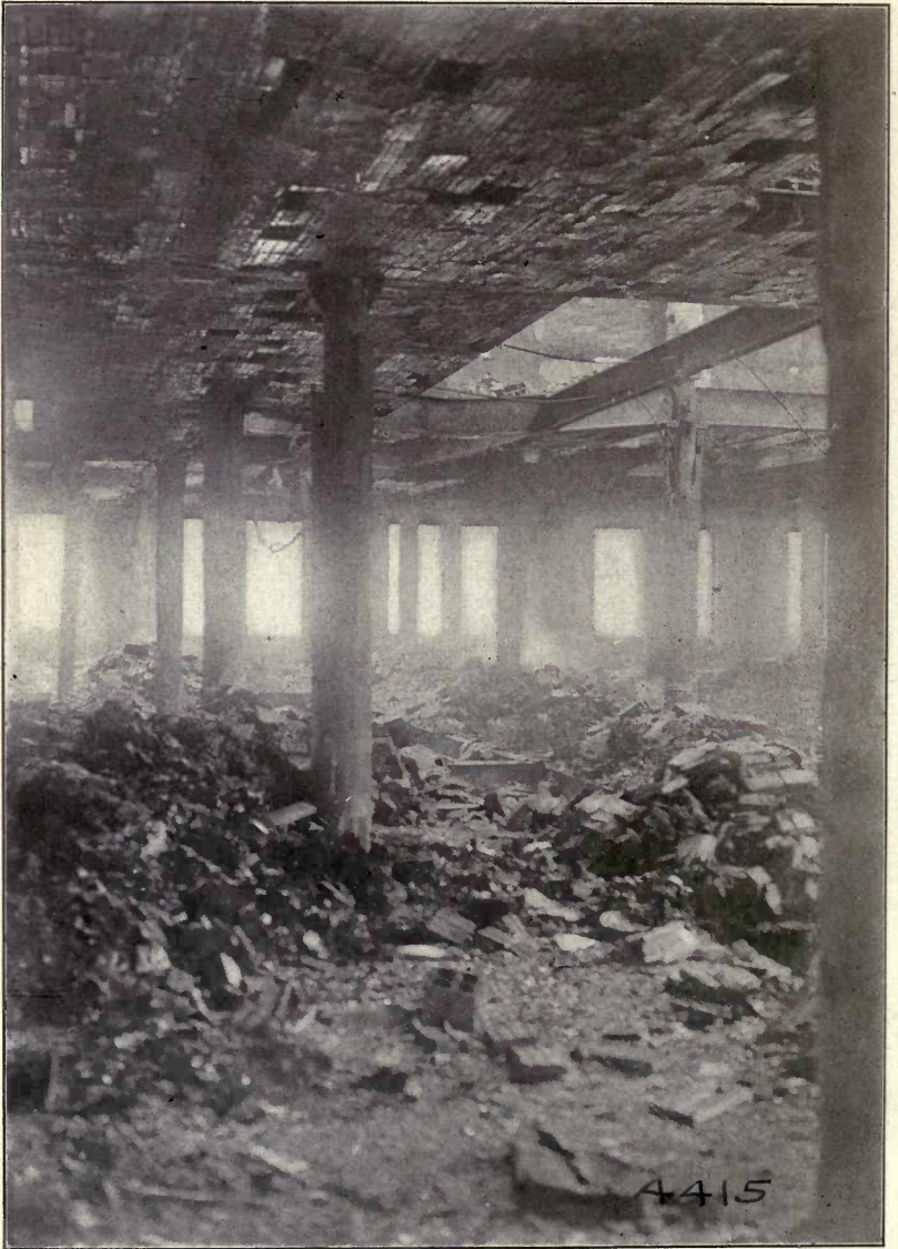
NINTH STORY, Looking North, Showing Damaged Soffits of Arches, Collapsed Arches, Deflected Beams, Damaged Column Covering, etc.
