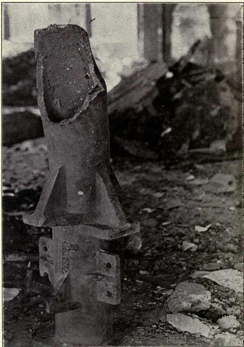
Collapsed Column (34 or 33), Eleventh Story, Showing Fracture and Effect of Heat. View Inverted.
