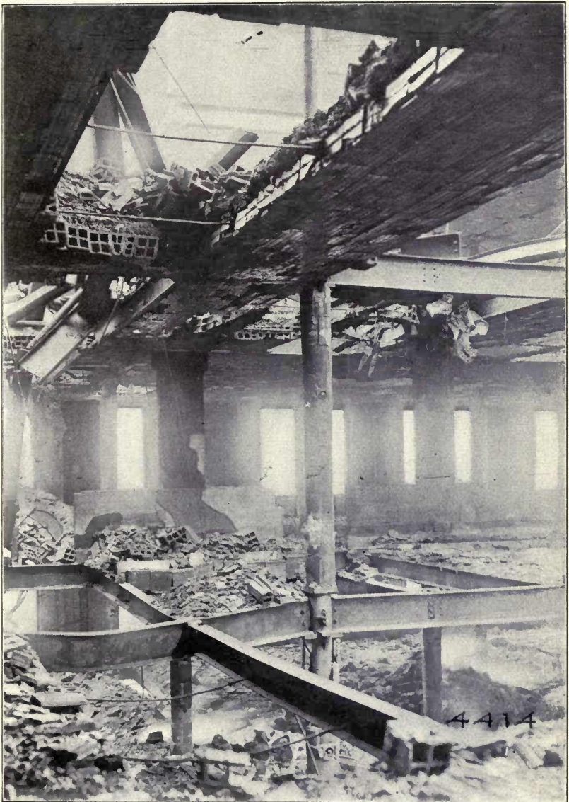
TENTH STORY, Looking North, Showing Damaged Beams, Collapsed Floor Arches, etc.
