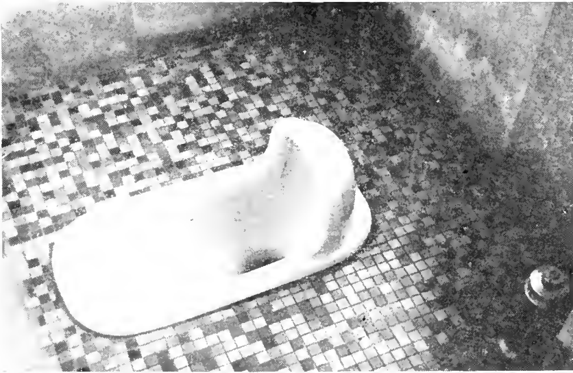
FIGURE 22. Vitrified china, squat type, toilet bowl with foot-operated flushing device, installed in modern office building, Tokyo.
