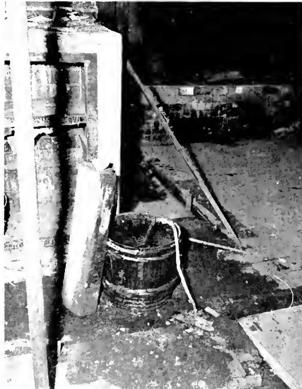
FIGURE 19. Leaking service pipe.
