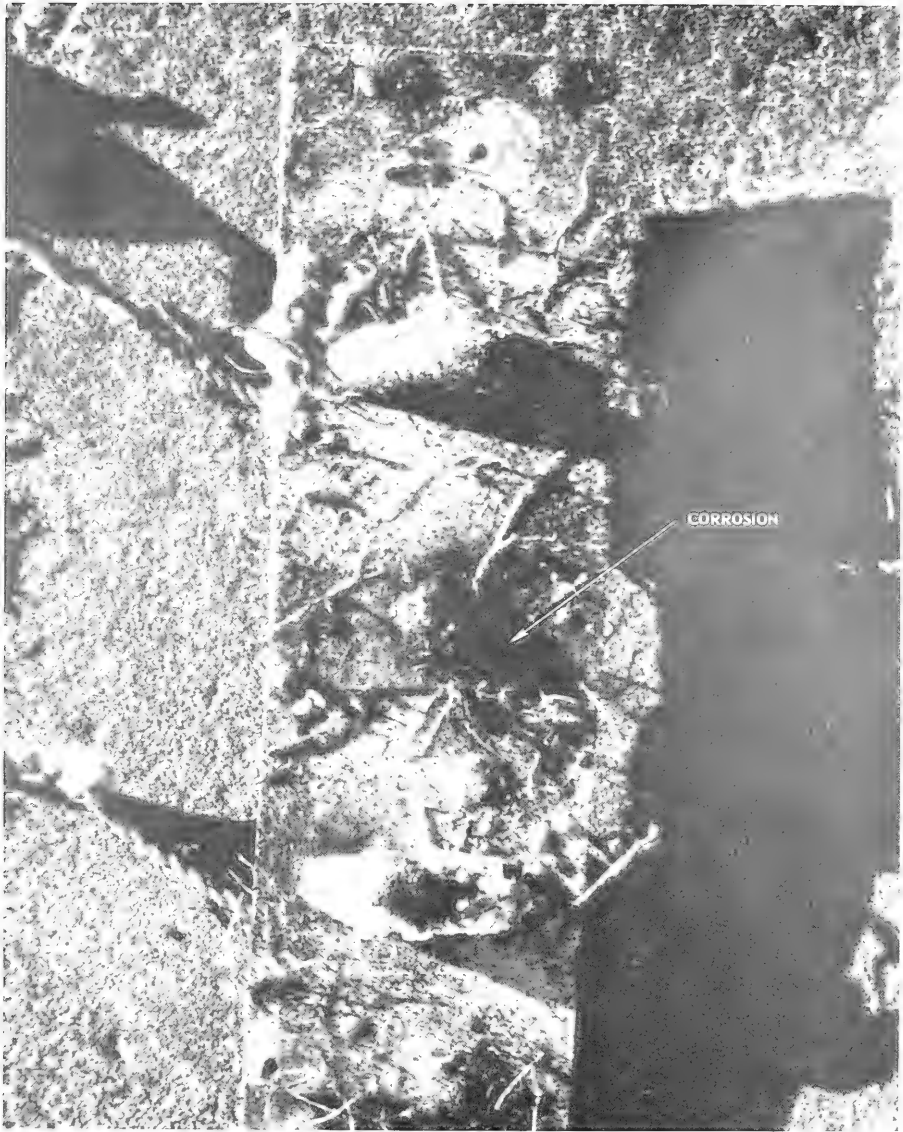
Figure 9. Corrosion-resistant steel panel (#8), uncoated, after submergence in SQUAW installation.
