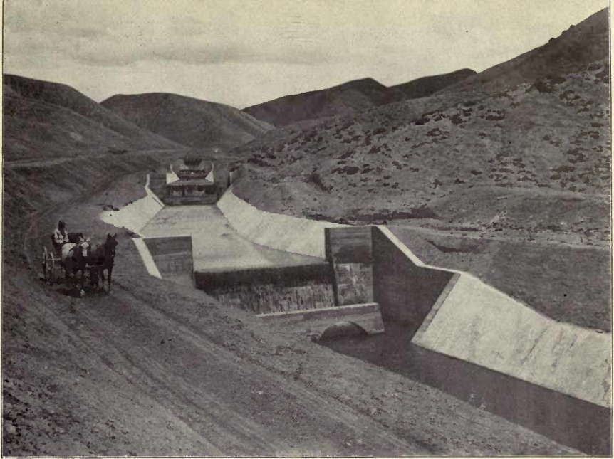
PL. IVA. Drops on South Canal, Uncompahgre project, Colo., taking otherwise useless Gunnison River waters to Uncompahgre Valley; method of dropping these waters to the Valley.
