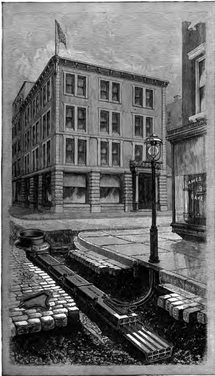
Johnstone Electric Conduit System.
