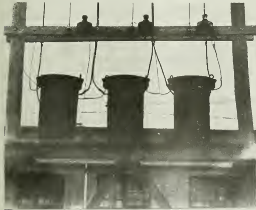
Fig. 1—Fuse cut-outs protecting pole type transformers.
