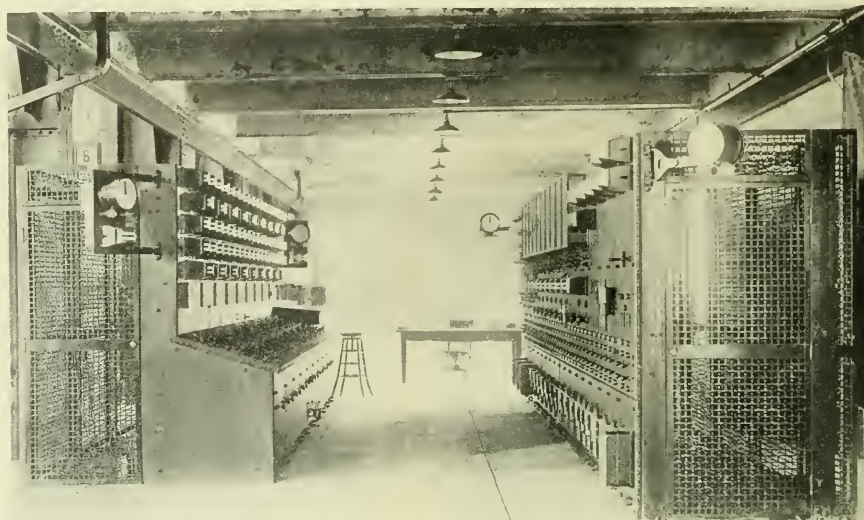
Power House Switchboard—Cedars Rapids Manufacturing and Power Co.
