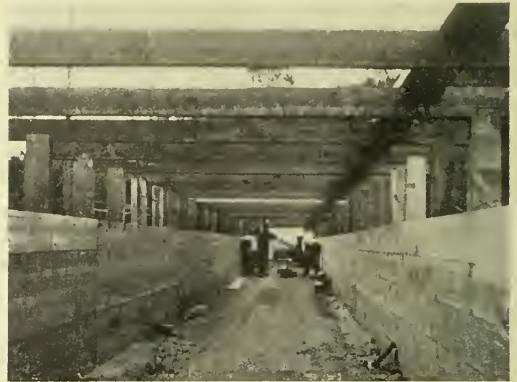
Fig. 5—Flume System, Hydro Plant—Kamloops, B. C.
