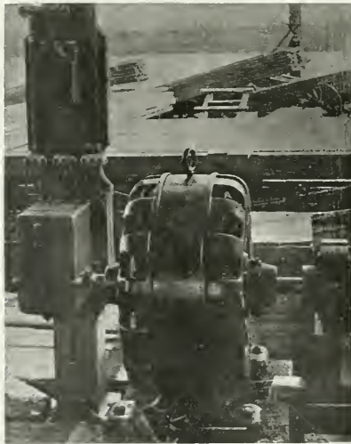
50 H.P. Motor Installation
