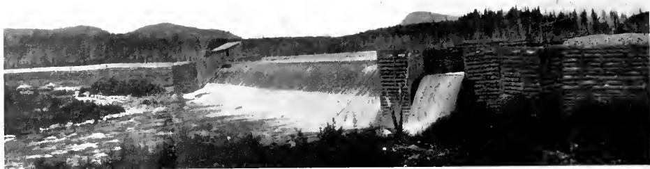
Storage Dam on Lake Omataway—An important part of the Price Bros. power development.
