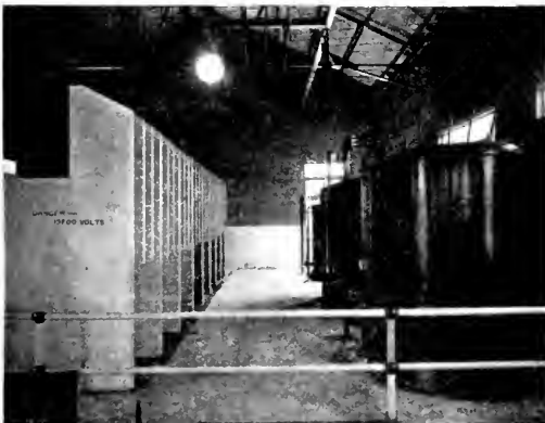
No. 8 Mine, showing sub-station transformers and high-tension switchgear in concrete cells.
