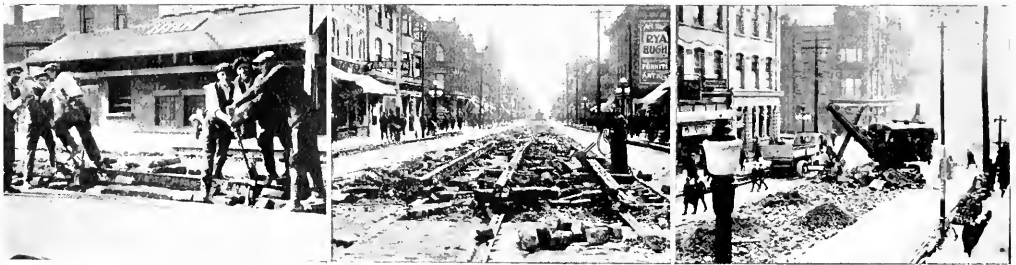
When a street car line is to be rehabilitated, the old rails are jacked up as shown in the left hand illustration and are then cut by means of an oxy-acetylene flame into lengths convenient for hauling to the storage yard. The granite sets or paving brick are salvaged, if of value, after which the grading of the road bed is carried out by means of a steam shovel, the spoil being carried away on motor trucks.
