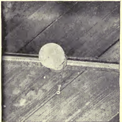
FIG. 27.—Surface metal raceway makes a neat job in an exposed location
