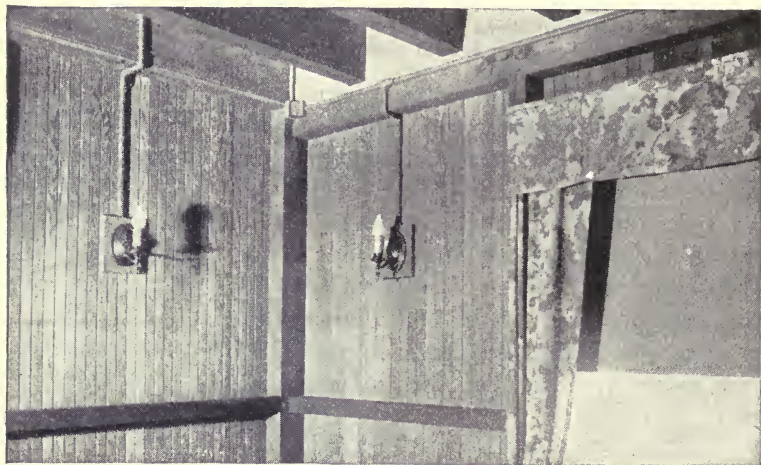
FIG. 90.—A Wiremold installation in a summer cottage
