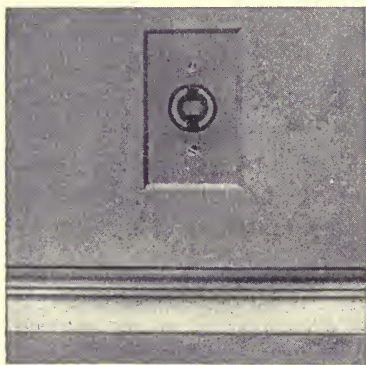
FIG. 14.—The single convenience outlet does not meet the requirements of an active room in the modern home
