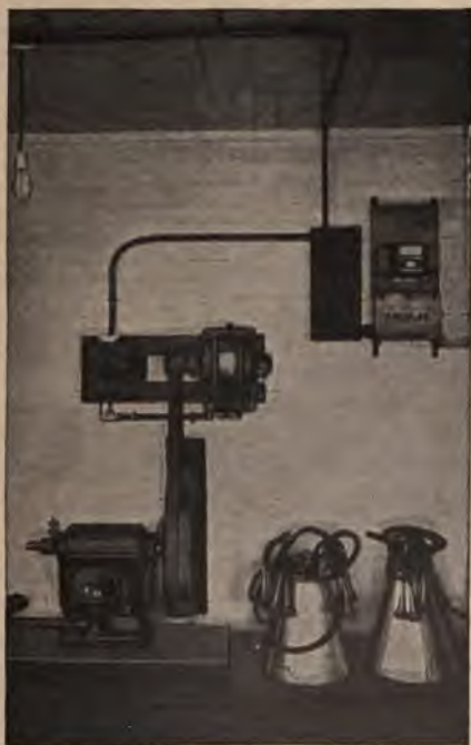
Fig. 35. Motor-operated (belt-connected) vacuum pump and milking outfit. The motor is mounted on the wall.
