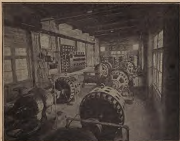
Fig. 51. Pumping plant of Snake River Irrigation Company's plant, southern Idaho. This plant irrigates approximately 15,000 acres. The equipment consists of one 30, two 20 and two 16-inch centrifugal pumps, lifting the water 57, 108 and 145 feet, respectively. Another pumping plant of this company irrigates 48,000 acres.
