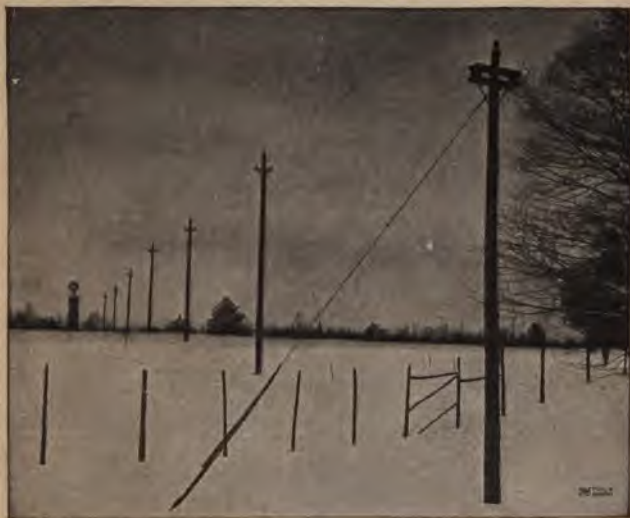
Fig. 7. Electric power transmission system on a New York farm.
