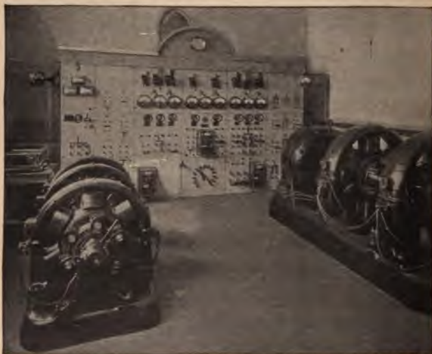
Fig. 1. Interior of the electric sub-station at a New York farm, showing motor-generator sets and switchboard.
