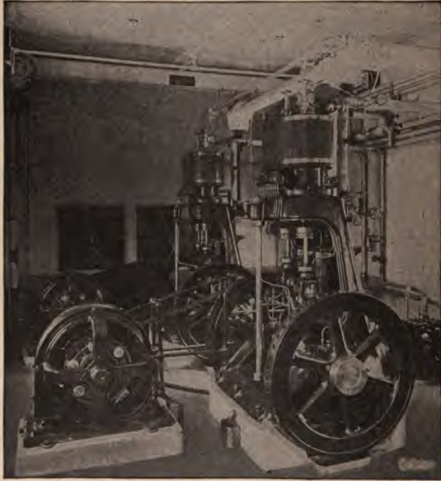
Fig. 24. Motor-operated ammonia pumps (chain connected) in ice-making plant on a New York farm.
