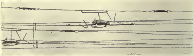
Yard section breakers with simple insulation. Messenger insulator removed from arcing region for protection
