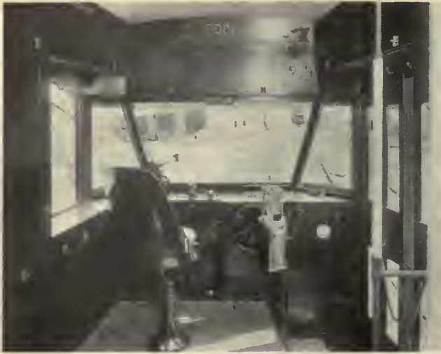
All apparatus in the front vestibule is inclosed in cabinets. Liberal door space permits easy access for inspection and repair. The control switch groups are in the cabinets at the left
