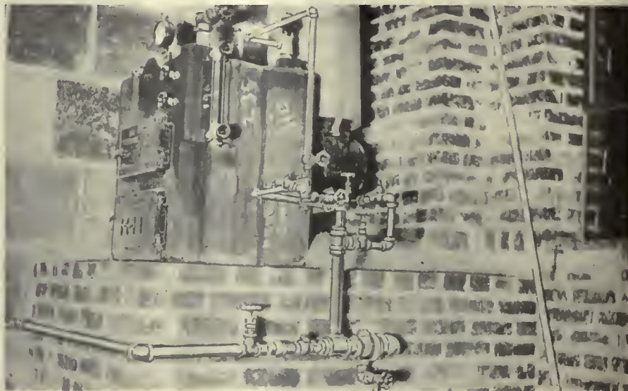
Portion of incinerator with automatic water-feed control
