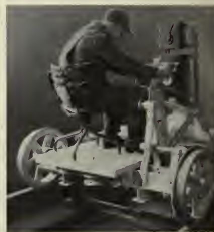
The operator's position has been chosen carefully to give a good view of the action of the tamping arms
