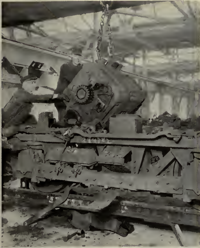
Workmen guide the motor so that the motor axle suspension seats properly as the motor is handled by an overhead crane
