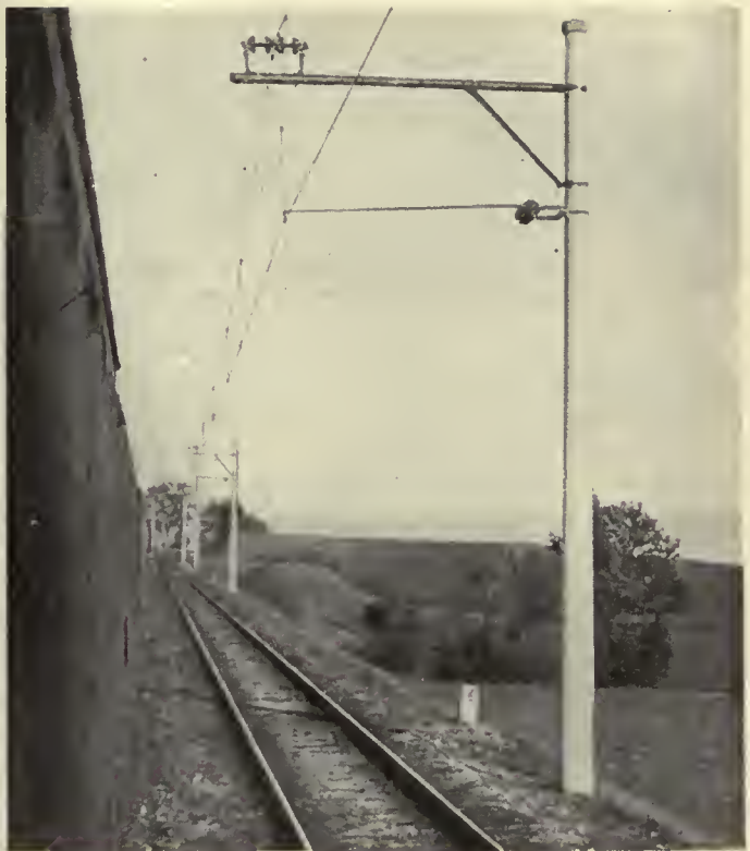
Single-track line showing use of concrete poles
