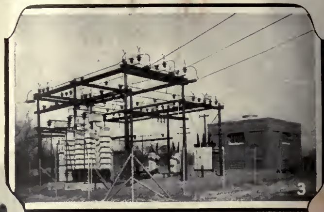
1.—Control panels, starting and running panels, and load-limiting resistance
