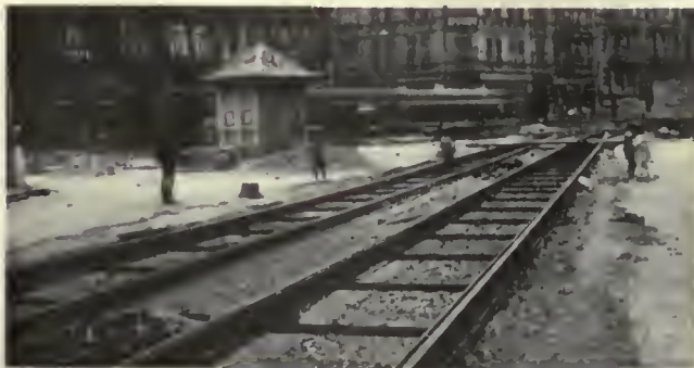
Fig. 10—Tangent track on concrete base with resilient filler and tie rods, before the installation of paving
