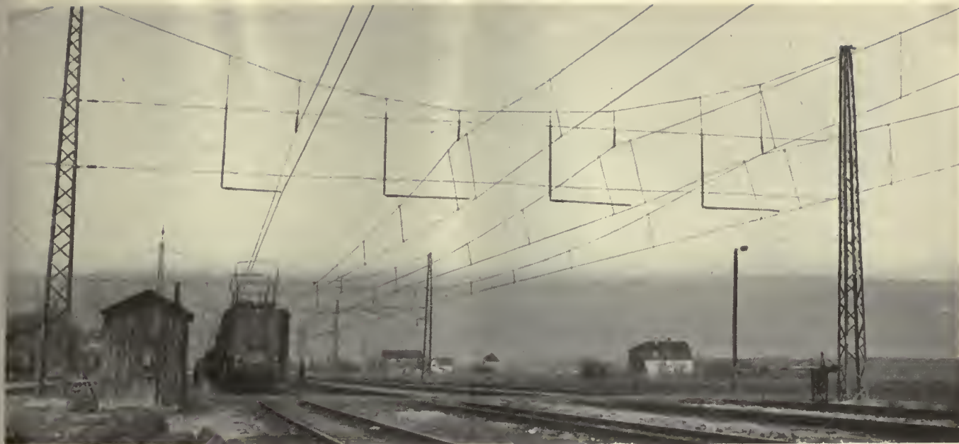
Latest type yard construction in Bavaria, with simple insulation, grounded cross-spans and track isolation
