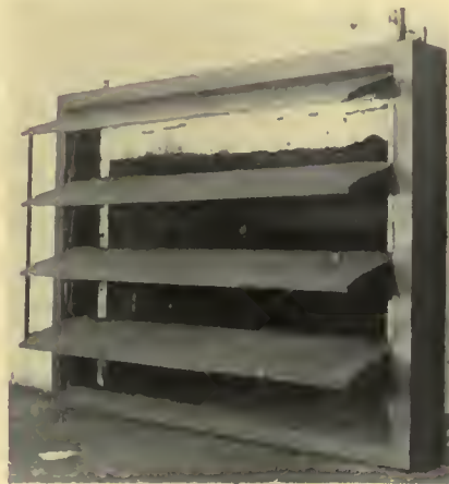
Fan shutter open in air chamber at Front Street substation of Toronto Transportation Commission
