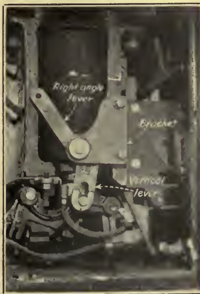
Device mounted on sectionalizing switch by which it is possible mechanically to close the contactor
