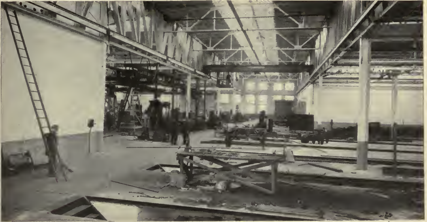
View of the pit room and the craneway. At the left of the crane are the armature repair and machine shops, and to the rear of these shops is the general storeroom
