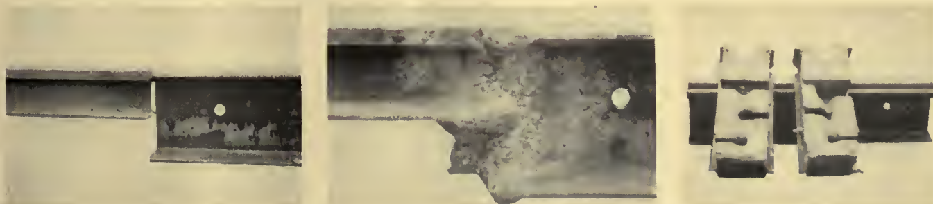
At left—80-lb. A.S.C.E. tee rail set up with 134-lb. girder groove rail. In center—Finished thermit weld. At right—A pair of mold boxes cut out and ready for applying to the joints
