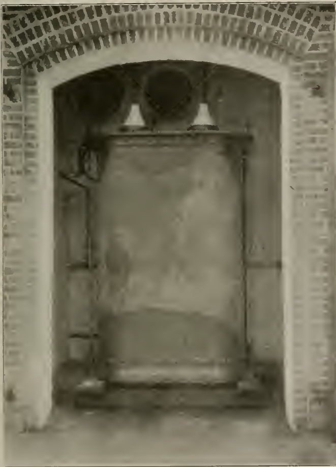
Portland Railway—Transformer Compartment with Entrance from Outside of Building.
