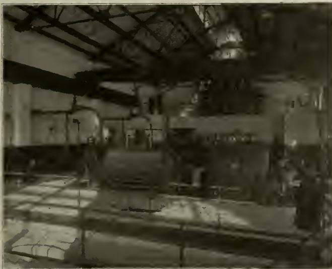
Pittsburg & Butler Street Railway—Turbine Room.
