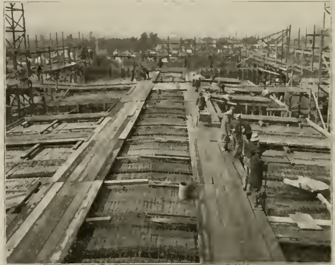
Seattle Electric Power Station—Roof During Construction, Showing Reinforcement and Cable Way for Handling Concrete.
