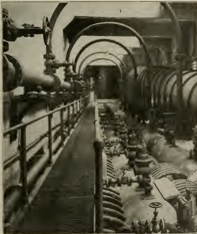
Seattle Electric Power Station—View of Boiler, Showing Facilities for Repairs and Inspection.
