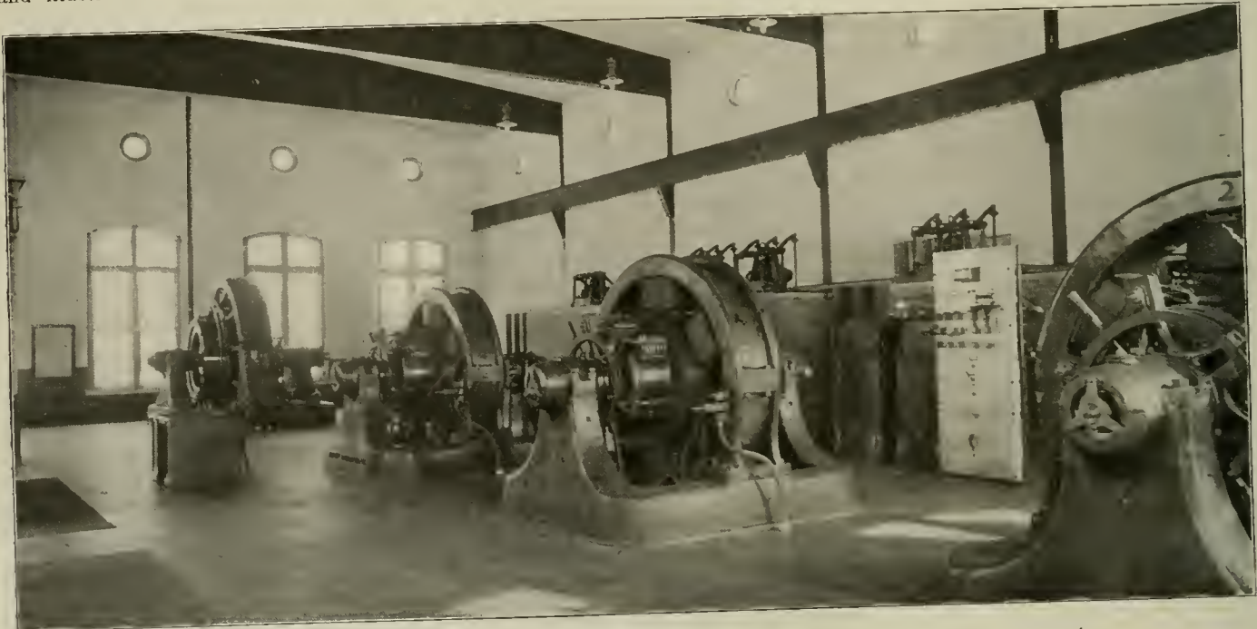
Seneca Street Substation, Buffalo—Interior View Showing 1,000-Kw. Rotary and Three 400-Kw. Rotaries.
