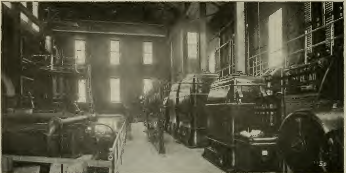
Philadelphia & Western—Interior of Power House, Showing Curtis Turbines, Switchboard and Transformers.
