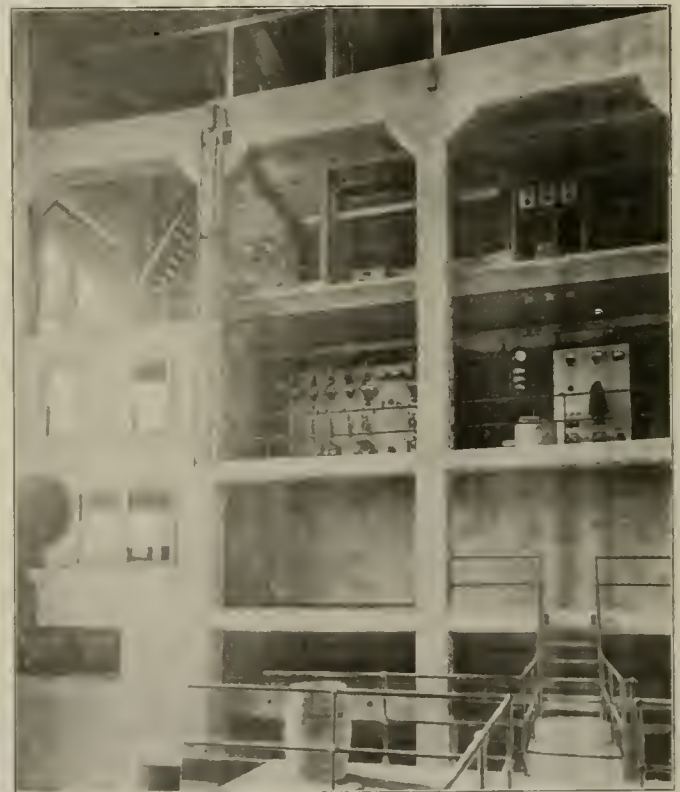
Seattle Electric Power Station—Interior of Engine Room, Showing Switchboard Galleries, Engineer's Office and Wash Room.
