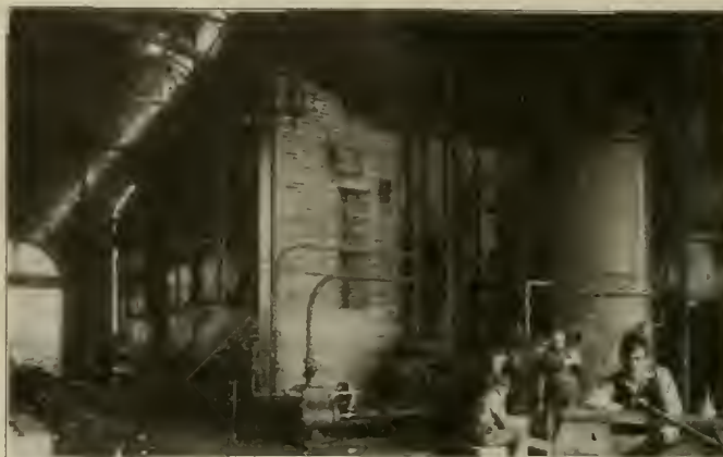
Pittsburg & Butler Street Railway—Boiler Room.
