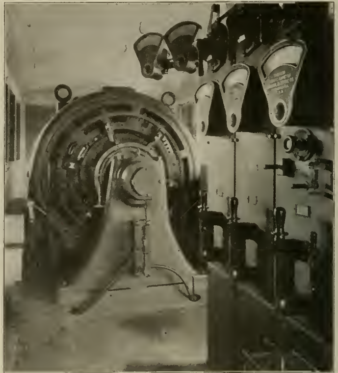
Northern Electric Railway—Interior of 60,000-Volt Portable Substation.
