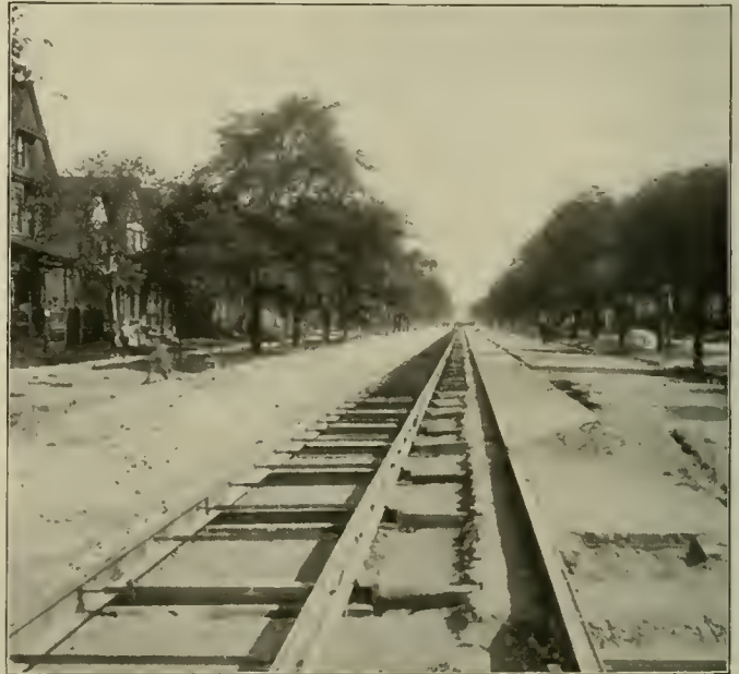
Track Construction with Nine-Inch Rails, Carnegie Steel Ties and Tie-Rods at Five-Foot Centers.
