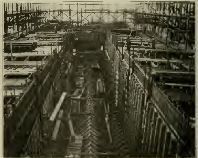
Seattle Electric Power Station—Coal Bunkers During Construction, Showing Method of Constructing Forms.
