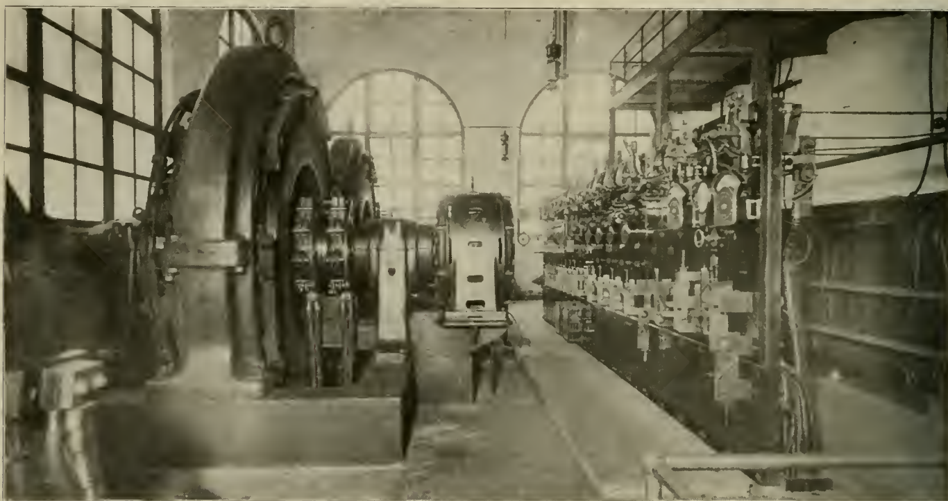
Metropolitan Elevated Railway—Interior Forty-Sixth Avenue Substation.
