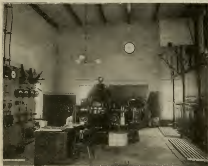
Pittsburg & Butler Street Railway—Interior View of Rotary Substation.
