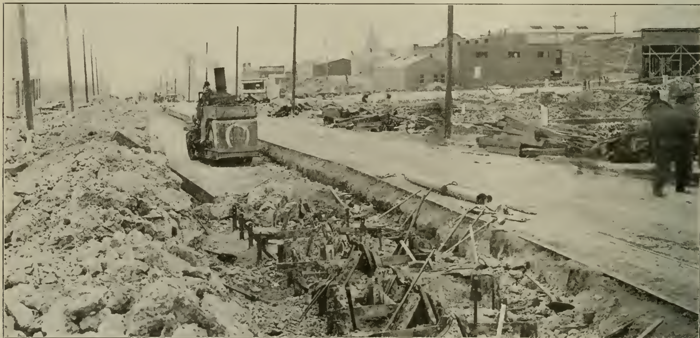
San Francisco Track—Breaking Off Old Cable Yokes and Rolling Bed for New Track.
