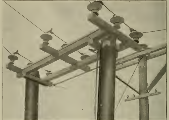
Open-Air High-Tension Switch.
