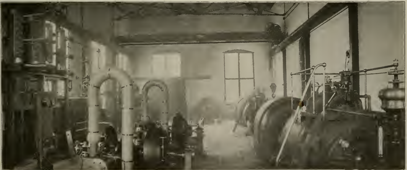
Ft. Dodge Des Moines & Southern Railway—Interior of Engine Room.
