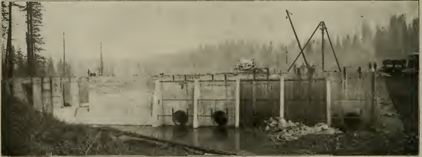
Cazadero Station of the Portland Railway—Forebay Wall and Penstock Openings During Construction.
