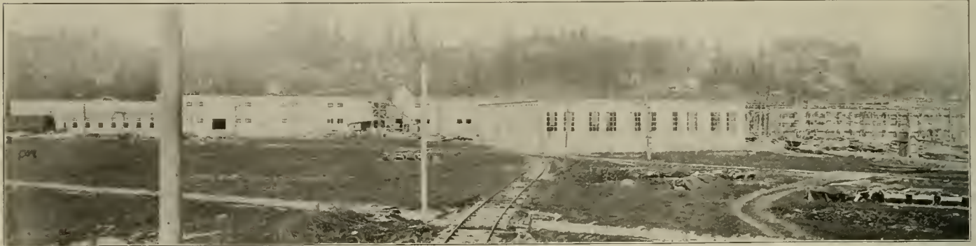
New Shops at Seattle—General View of Buildings During Construction—Store Room at the Left, Paint Shop at the Center, Erection Shop at the Right.
