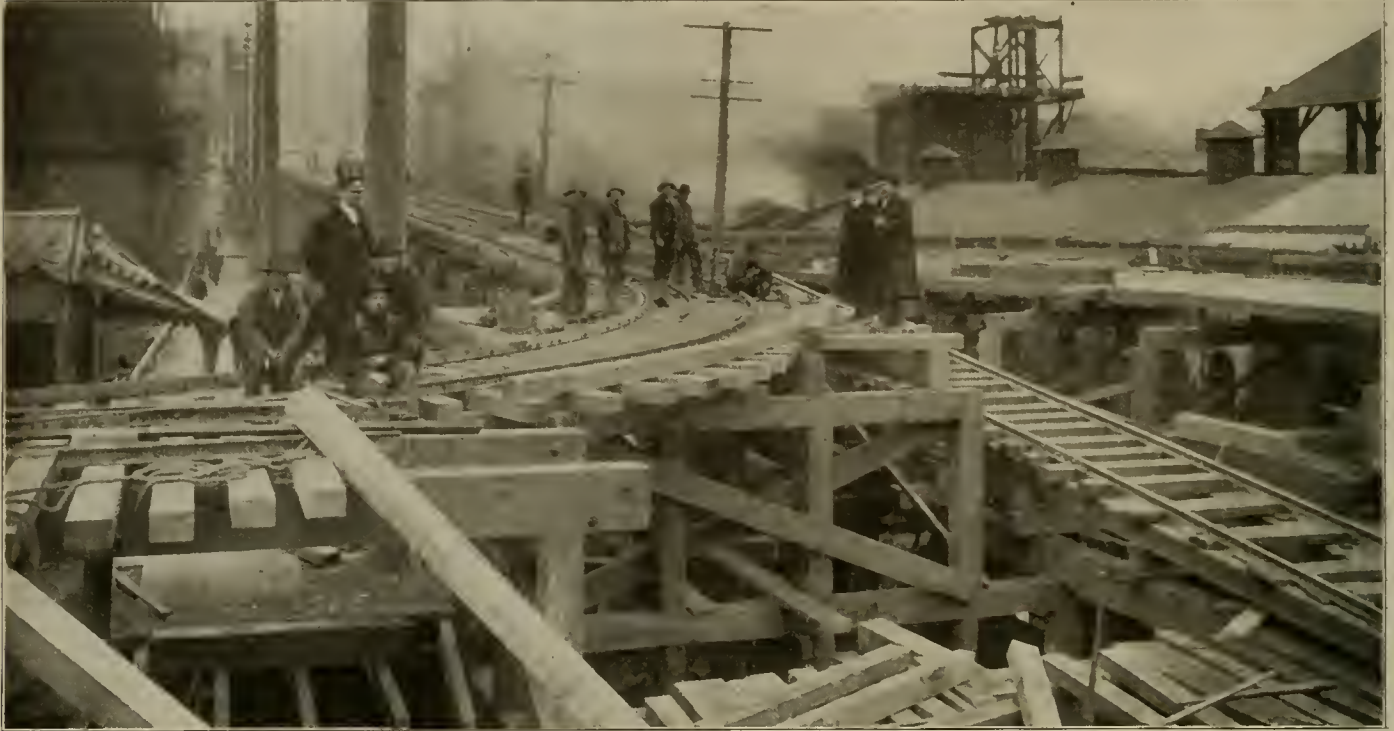
Adjusting Grades in Seattle—Blocking Up Track 17 Feet Prior to Raising Street Grade.
