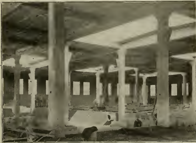
New Shops at Seattle—View of Incompleted Interior of Machine Shop, Showing Sunken Floor over Which Will Be Placed Repair Tracks.
