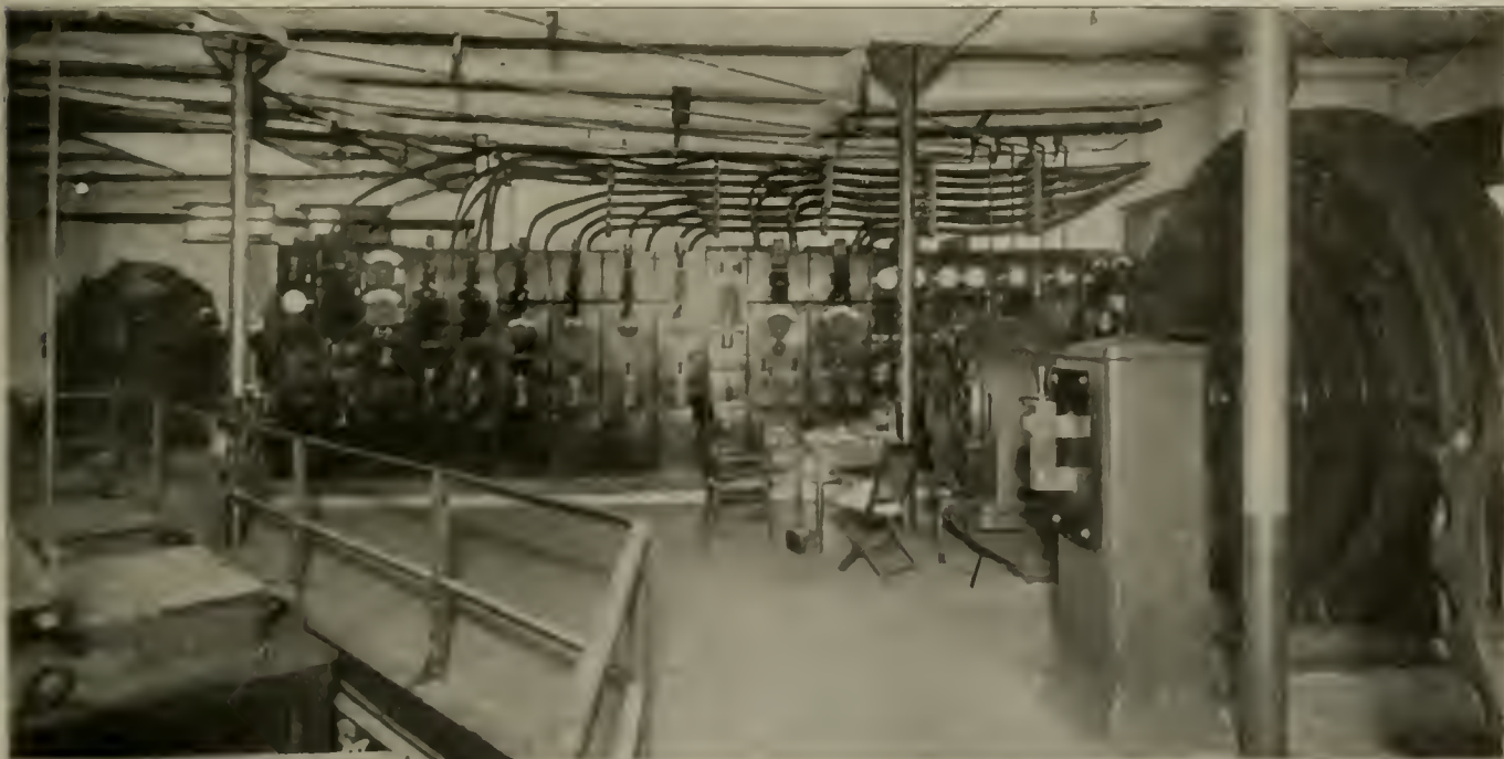
Metropolitan Elevated Railway—Interior Robey Street Substation.
