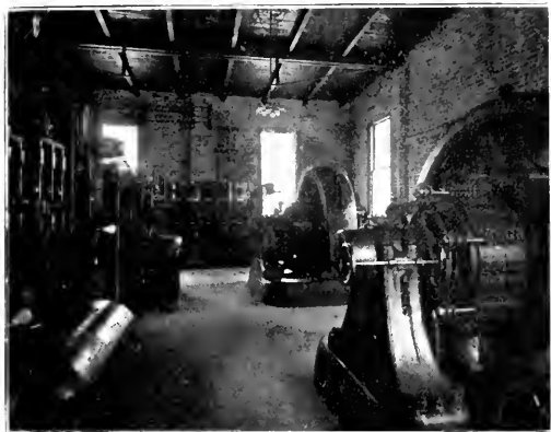
Chicago & Southern—Interior Blue Island Substation.
