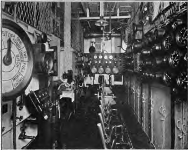
FIG. 119.—U. S. S. Tennessee : Assembly of Main Switchboard and Operating Levers
