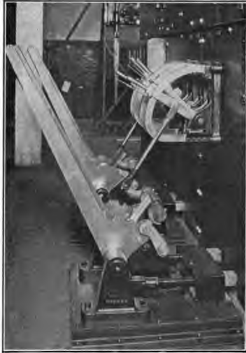
FIG. 74.—U. S. S. New Mexico : Main Switchboard, Partial View of Control Levers
