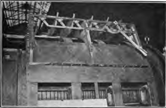
FIG. 84.—U. S. S. California : View of Alternator Showing Air Discharge Damper
