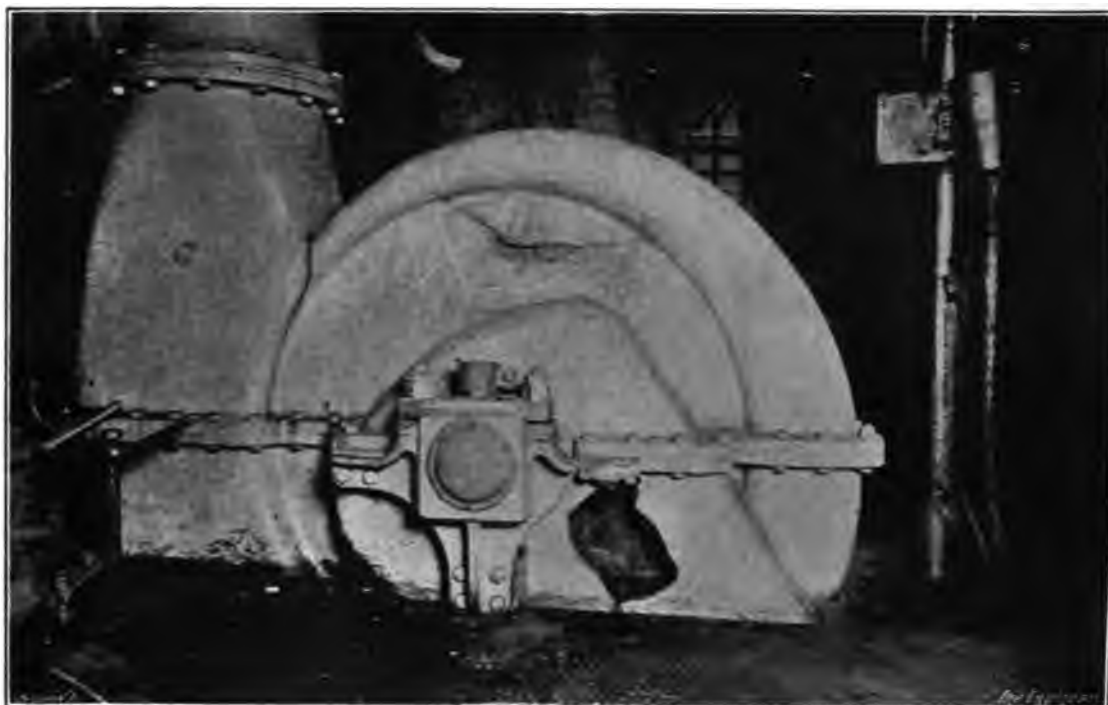
FIG. 73.—S.S. George Washington —Fractured Circulating-Pump Casing.
