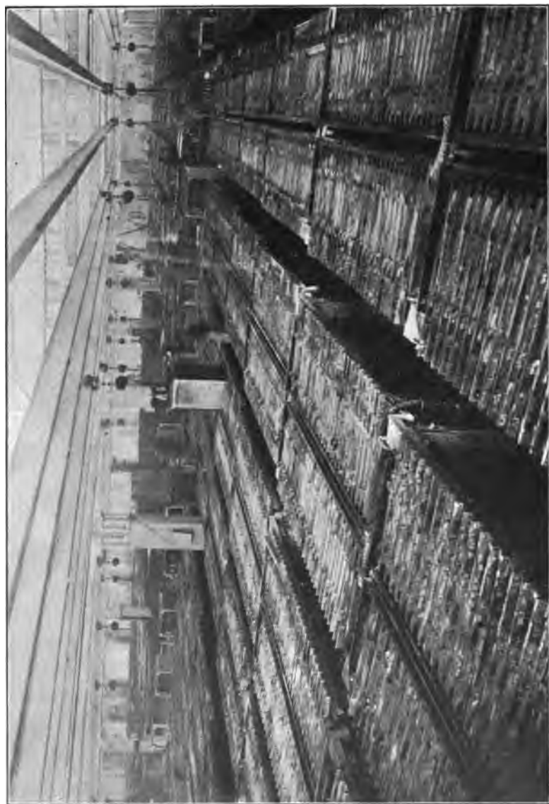
Cell Room in Zinc Plant at Great Falls, Montana
