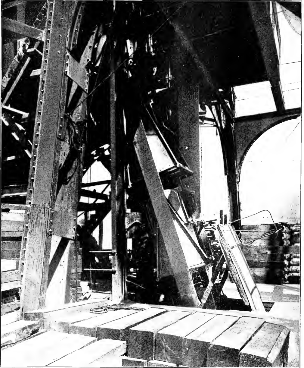
HIGHLY DEVELOPED HOISTING METHODS AND APPARATUS AT BUTTE, MONT. Illustration shows the cage- and skip-changing device of a modern hoisting plant
