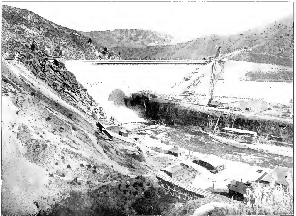
THE ARROWROCK DAM, NEAR BOISE, IDAHO; THE HIGHEST DAM IN THE WORLD. Construction was completed on Oct. 4, 1915. It is on the Boise project of the United States Reclamation Service, is 348.5 ft. above bedrock and 250 ft. above river bed. About 530,000 cu.yd. of cyclopan concrete was used.
