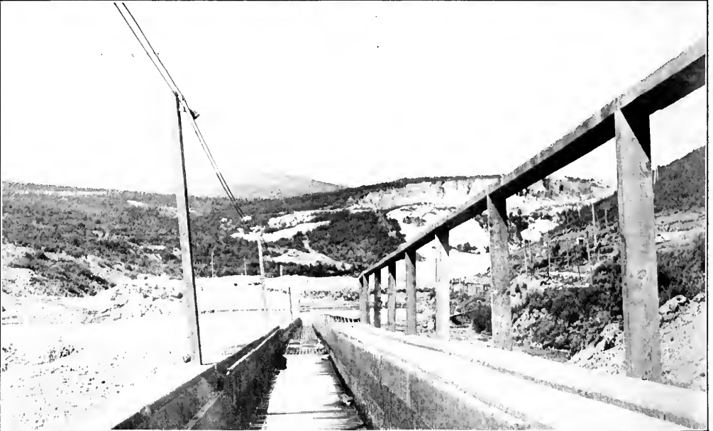
CLEANING BEDROCK AT ELEVATOR NO. 3. PREVIOUS TO THE APPLICATION OF DREDGING THE BONANZA CREEK GRAVELS WERE HANDLED BY HYDRAULICKING IN CONNECTION WITH MECHANICAL ELEVATORS. LOWER VIEW SHOWS THE UPPER SLUICE OF ELEVATOR NO. 3
