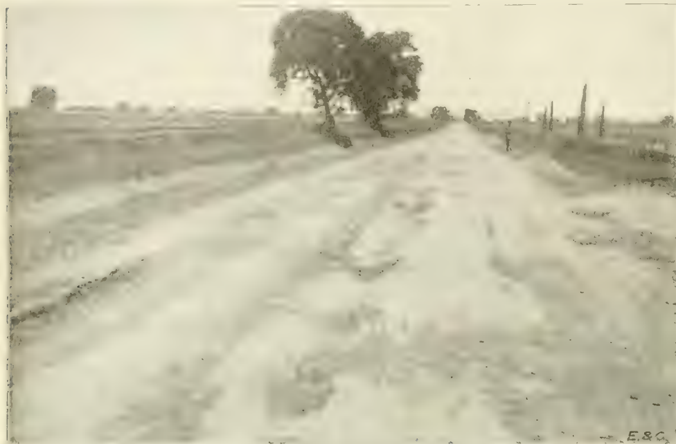
Fig. 8. Surface Failure on a Wet Adobe Foundation.
