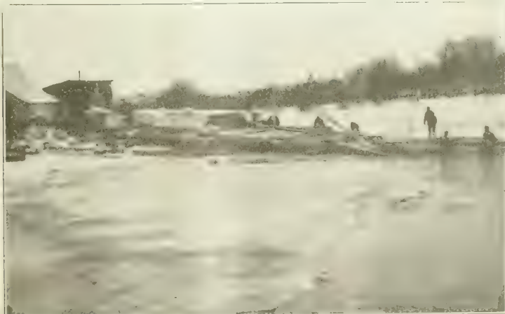
Fig. 5. View Showing Launching of Shoe of Caisson for Intermediate Pier—Richelieu River Bridge.
