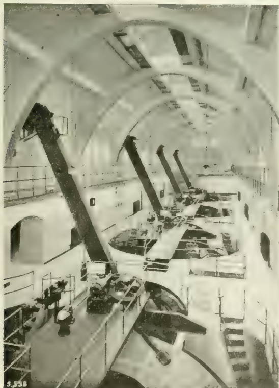
Fig. 6. Interior View of the Sewage Treatment Plant at Dresden, Comprising Four Riensch-Wurl Screens Each 26 ft. in Diameter.
