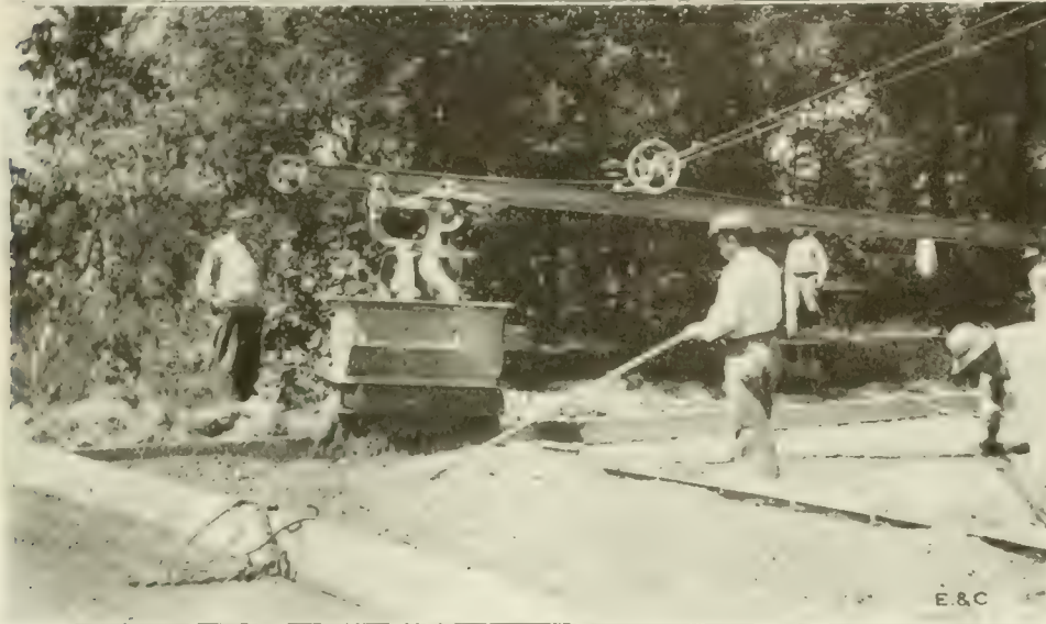
Fig. 4. Side Forms and Expansion Joint in Place. Striking Board in the Foreground.
