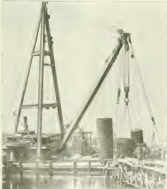
Fig. 6. View Showing the Placing of the Steel Encased Section of Chelsea Shaft for the Chelsea Creek Water Tunnel, June, 1914.
