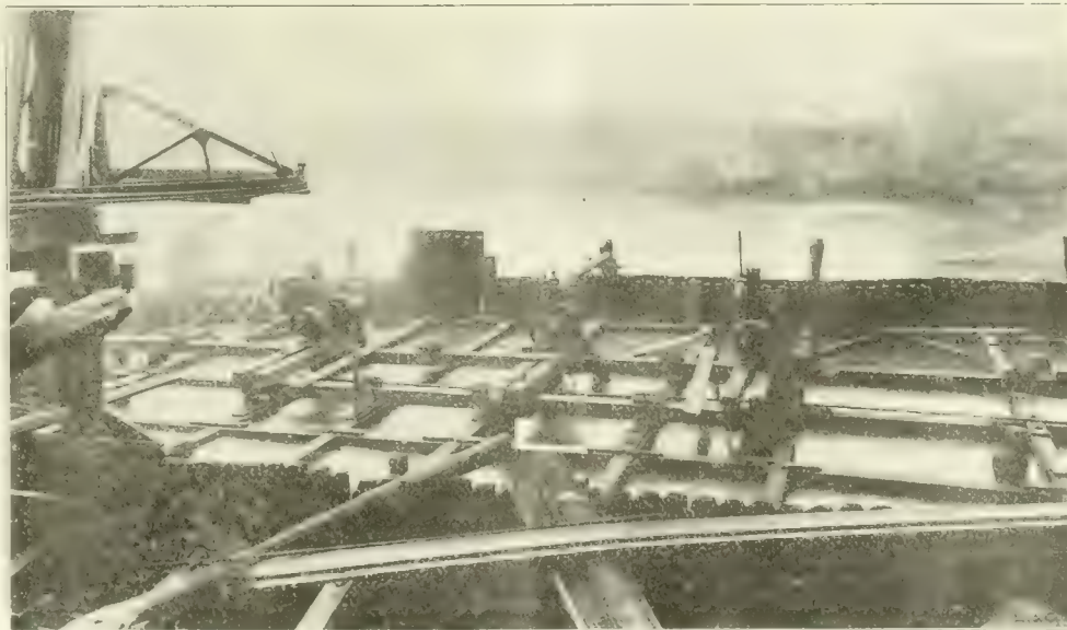
Fig. 6. View from Northeast of East Cofferdam for Chicago Ave. Bridge, Showing Top Tier of Bracing and Centrifugal Pumps in Place—Raised Section of Sheeting Is Over Water Pipe Tunnel.
