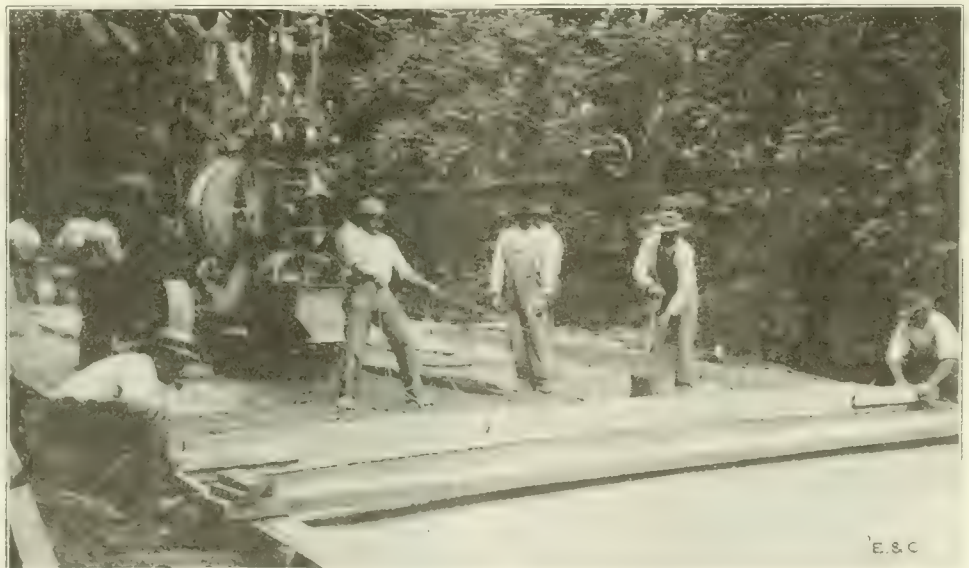
Fig. 3. Construction in Progress Showing Method of Handling Striking Board and Mixing Plant.
