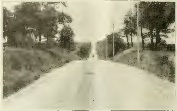
Fig. 4. Completed Road Surface. The Shoulders and Ditches of the Old Road Undisturbed.
