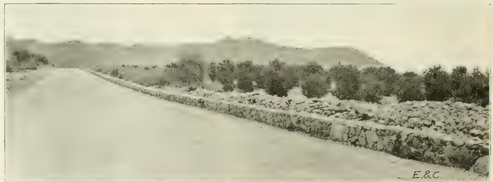
Fig. 5. View Showing Surface of Foothill Boulevard After Four Years of Service.
