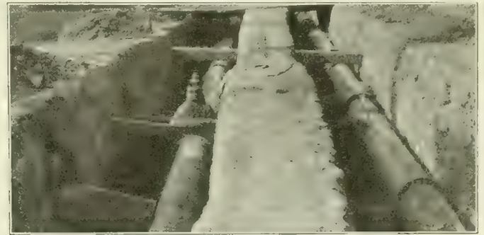
Fig. 2. View of Parallel High and Low Service Mains Ready for Lowering Under Pressure. Note Supporting Sections of Earth Back of Each Bell.
