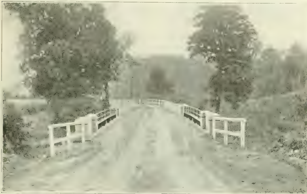
Fig. 4. View Showing a Brick Surfaced Highway. Note Guard Rail and Hand Rail on the Plate Girder Bridge.
