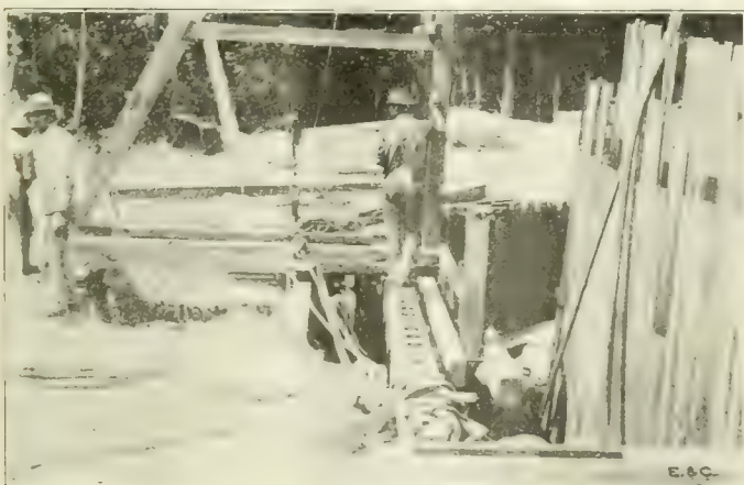
Fig. 2. View of Driving of 6 in. Sheet Piling in Sinking Large Dug Well in Water Bearing Sand at Atlantic City.
