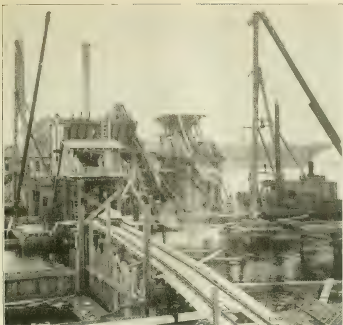
Fig. 8. View of Concrete Mixing Plant and Equipment Used in Mixing and Placing Concrete—Larz Anderson Bridge.
