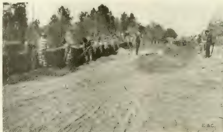
Fig. 7. Securing Clay by Digging Trenches at the Side of Road and Spreading Over Sand Bed in Center of Roadway.
