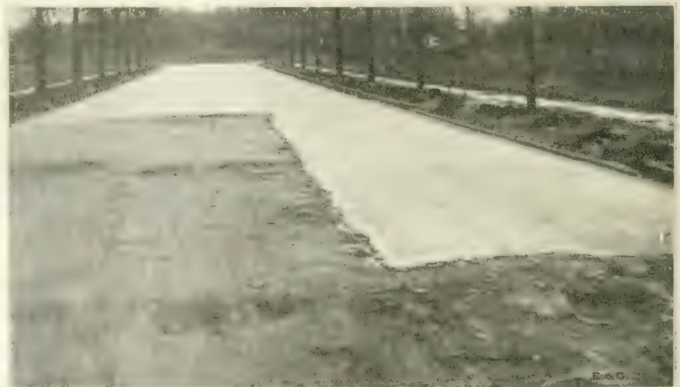
Fig. 3. Typical Resurfacing. Surface Prepared by the Heater in the Foreground, New Material Added and Finished Surface in the Background.
