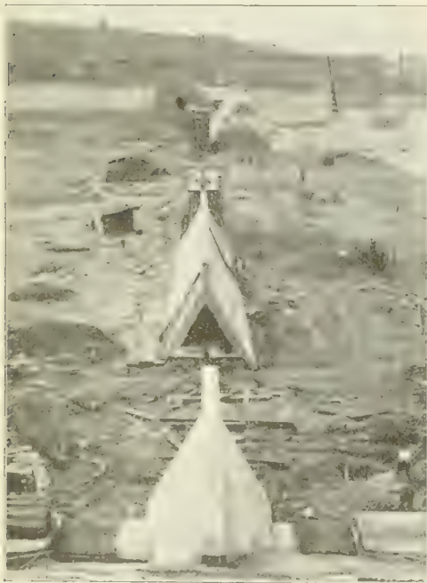
Fig. 1. View of Combined Dividing Wall and Inlet Conduit of North Side Reservoir, of Pittsburgh, Under Construction.
