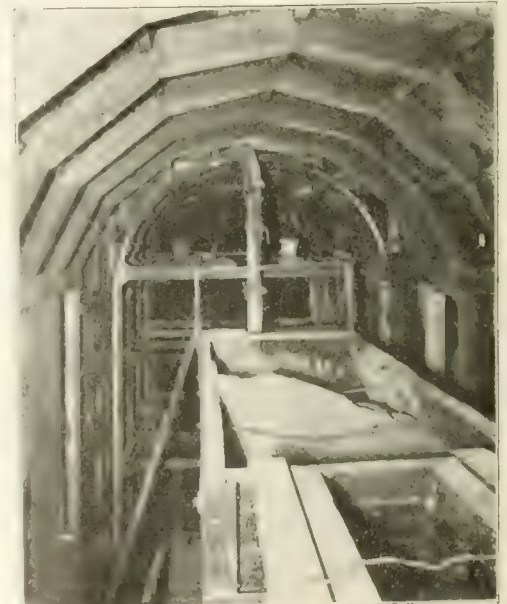
Fig. 3. View Looking Through Steel Forms at Delivery End of Car During Concreting.
