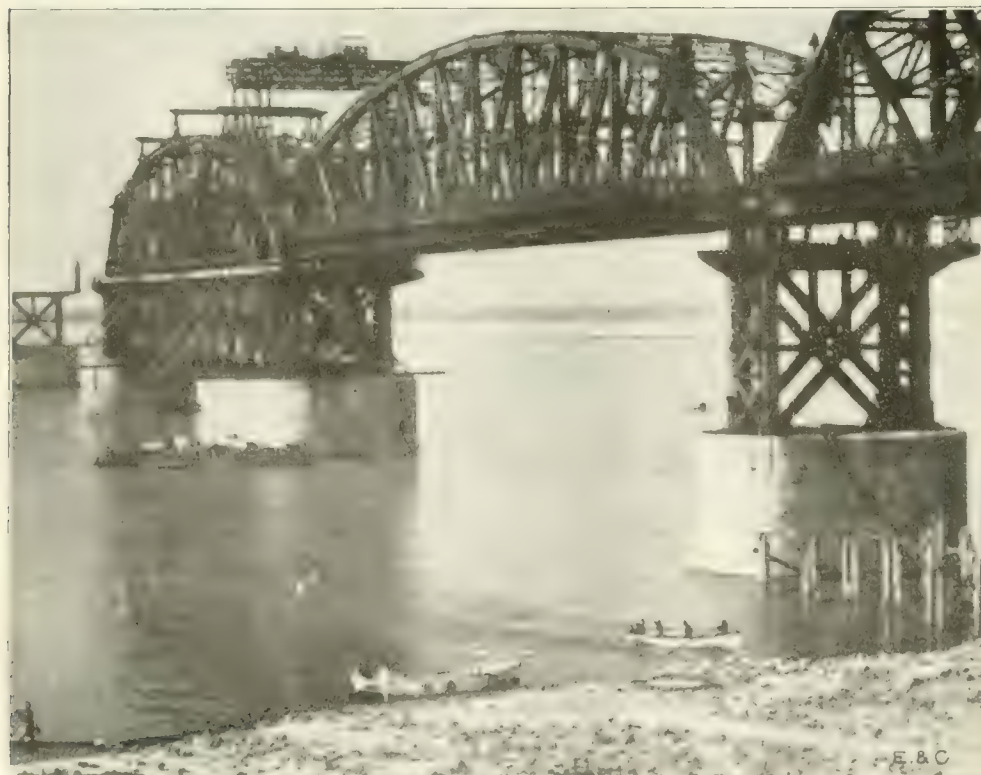
Fig. 7. View of Lower Ganges Bridge Showing Erection of a Main Span on the Erection Truss—View Also Shows a Completed Span and Pier.
