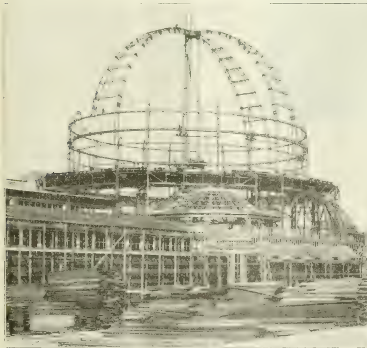
Fig. 18. View Showing Manner of Erecting Steel Framed Dome of Palace of Horticulture. View Also Shows Other Details of Building.
