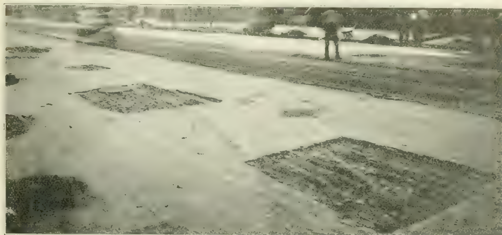
Fig. 4. Typical Patching Work on Wabash Avenue, Chicago, Showing Area Prepared for the Addition of New Material.
