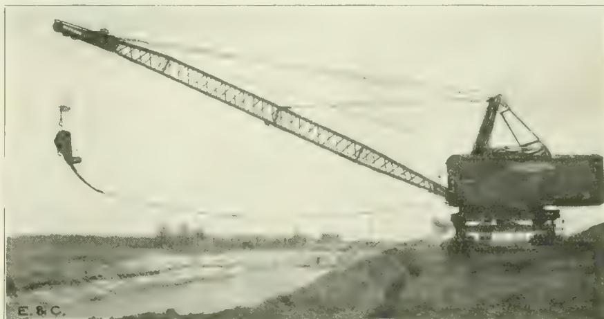
View of Largest Electric Dragline Excavator, at Work on Calumet-Sag Canal, Blue Island, Illinois.
