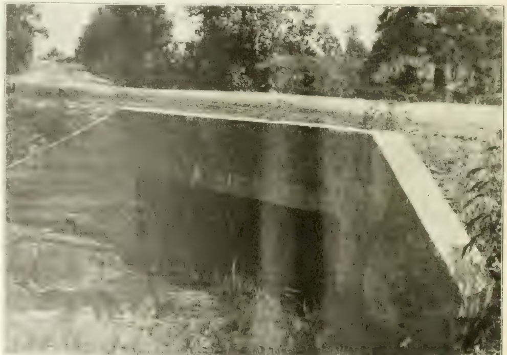
Fig. 2. View looking a Typical Concrete Culvert. The Bottom is Paved With Concrete.
