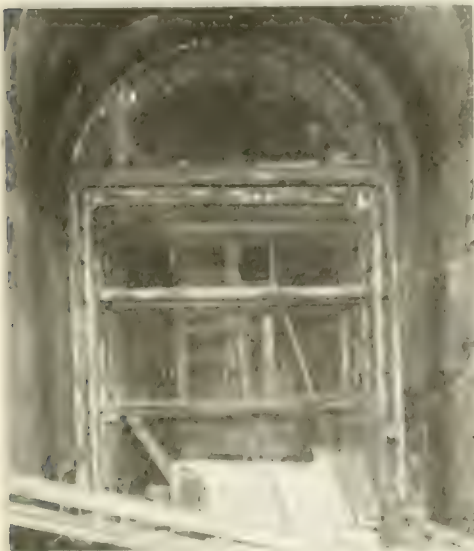
Fig. 2. View Showing Old Wooden Lining Blaw Forms, Concrete Delivery Pipe, and Top of Concreting Car, Burlington Tunnel at Arminto.
