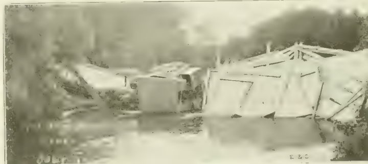
Fig. 2. View Showing Extent of Failure of Pony Trusses—Note That Load Did Not Break Through Floor.
