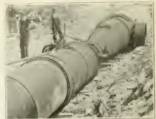
Fig. 10. View of Connection of 60 in. Cast Iron Pipe with 80 in. Steel Pipe, Weston Aqueduct Supply Main.
