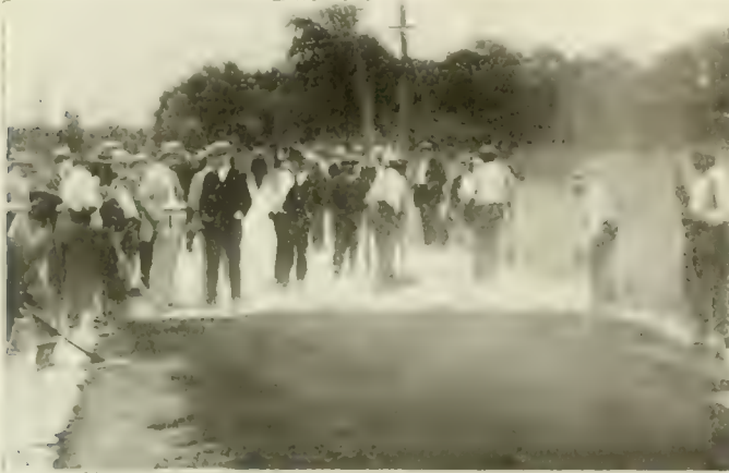
Fig. 3. Smoothing Bituminous Concrete Surface Prior to Rolling. Note Guide Boards at Sides.
