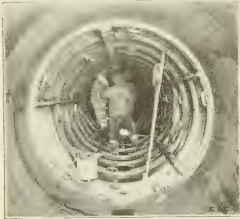
Fig. 9. View of Forms for Placing Mortar Lining of 80 in. Steel Pipe of Weston Aqueduct Supply Main.
