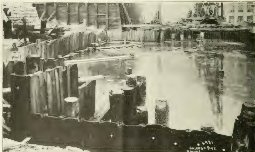
Fig. 4. View from South of West Cofferdam for Chicago Ave. Bridge—Note Two Types of Sheeting and Brace Piles.
