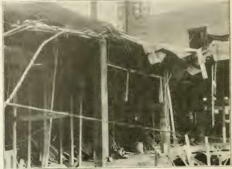
Fig. 3. View of Wrecked Portion of Theater and Arcade Building—Note Squareness of Girder Fracture—See Fig. 1 for Location of Camera.
