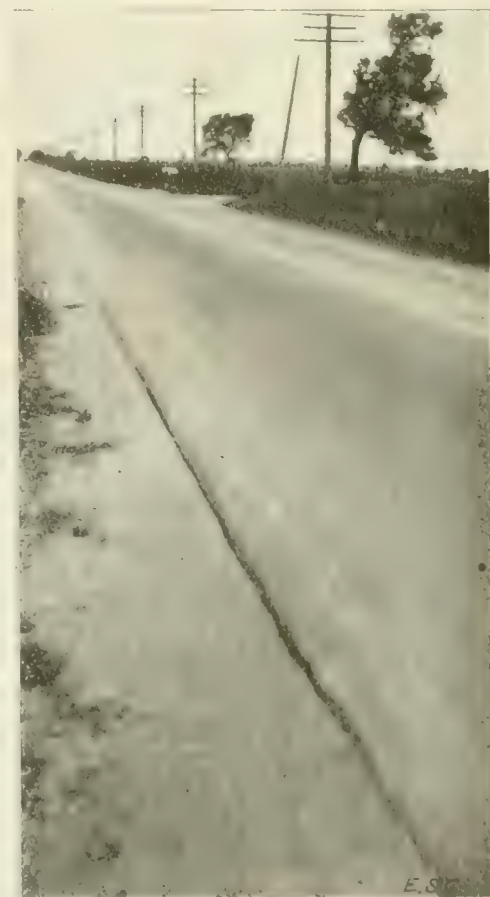
Fig. 10. Earth Shoulder Along Asphalt Macadam Pavement Worn Away by Traffic.
