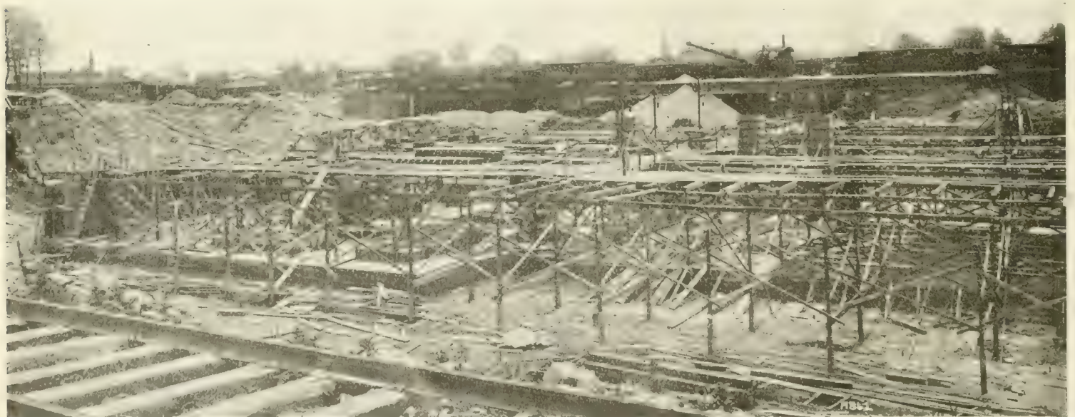
Fig. 3. View From North Showing East Half of Site of Detroit Station. Note Construction on Plant and Concrete Mat—Plant and Type of Construction for West Half Similar to That Shown in This View.
