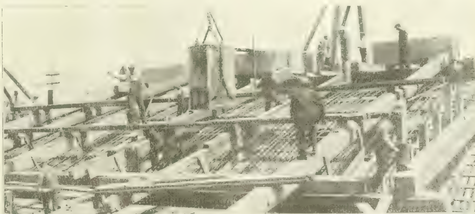
Fig. 11. View During Concreting of Arch Ring of Larz Anderson Bridge—Load at Crown Is About 25 Tons.
