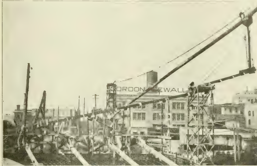
Fig. 8. View of Portion of Concrete Spouting System for San Jacinto St. Bridge. Note Wooden Distribution Spouts.
