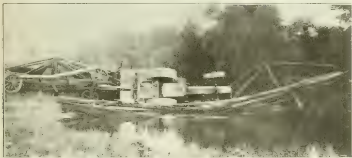
Fig. 1. View of Highway Bridge Failure Near Albany, Wis.—Pony Trusses Pried Apart to Give Clearance to Truck Loaded With Forms.
