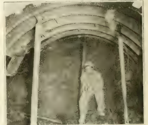
Fig. 8. View of Steel Roof Plates Used in Driving Extension to Mystic River Water Tunnel in 1912.
