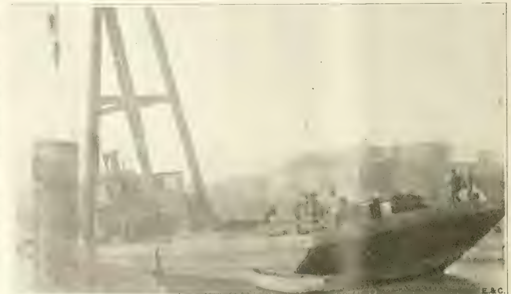
Fig. 9. View Showing the Pulling Up of the Old South Shaft of the Mystic River Water Tunnel.
