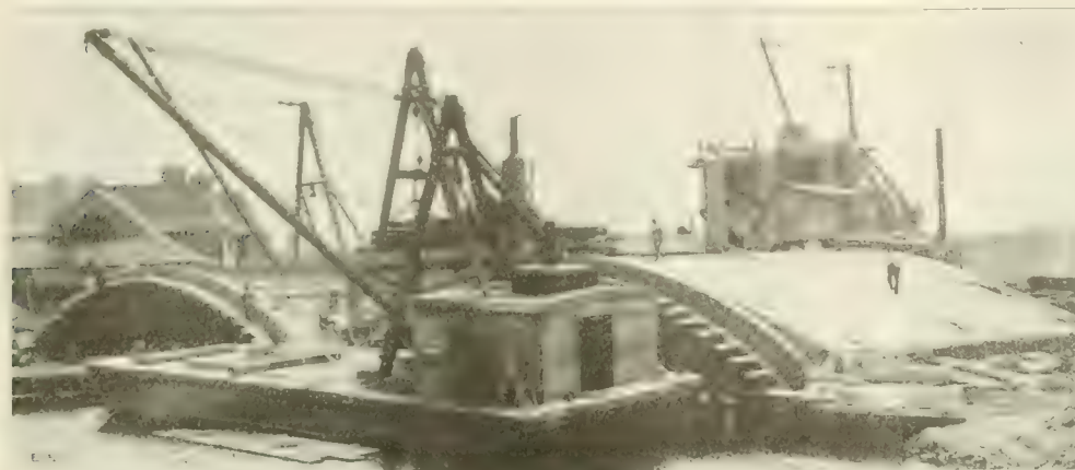
Fig. 12. View Showing Men Placing Reinforcement in Arch at Cambridge Side and Completed Arch Ring at Boston Side—Larz Anderson Bridge.
