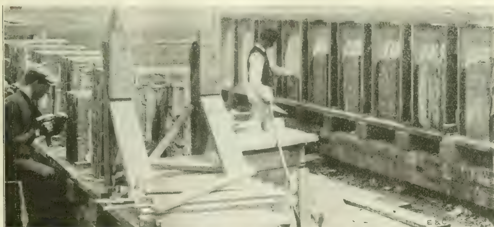
Fig. 10. View Showing Manner of Constructing Brick Voussoirs for Facing Ring of Arches of Larz Anderson Bridge.
