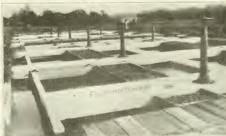
Fig. 5. View of Top of Moorestown Sewage Tank, Showing Floating Sludge.
