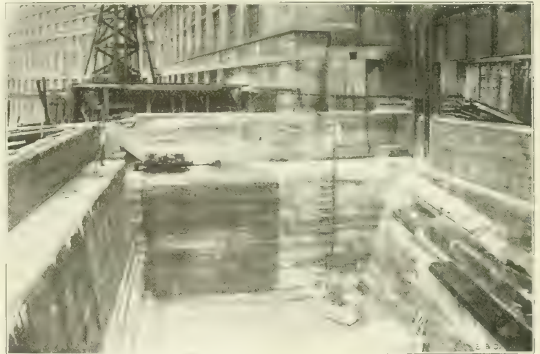
Fig. 8. View from South of East Piers and Pit of Chicago Ave. Bridge—Note Anchor Column and Floorbeam.
