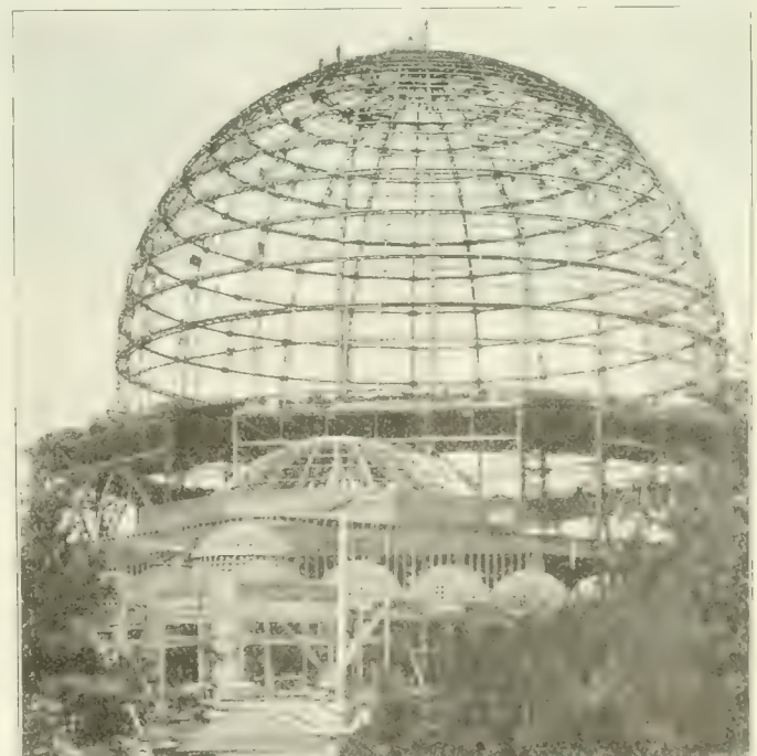
Fig. 19. View Showing Steel Frame of Dome and Its Supports, Palace of Horticulture.
