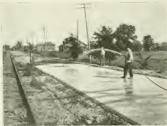
Fig. 5. Sprinkling Finished Road and Covering with Earth. Sprinkling Is Continued at Least 8 Days.
