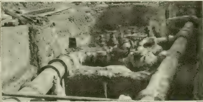
Fig. 1. View of Connection of High and Low Service Mains at San Diego, Calif, as Excavated for Lowering Under Pressure.
