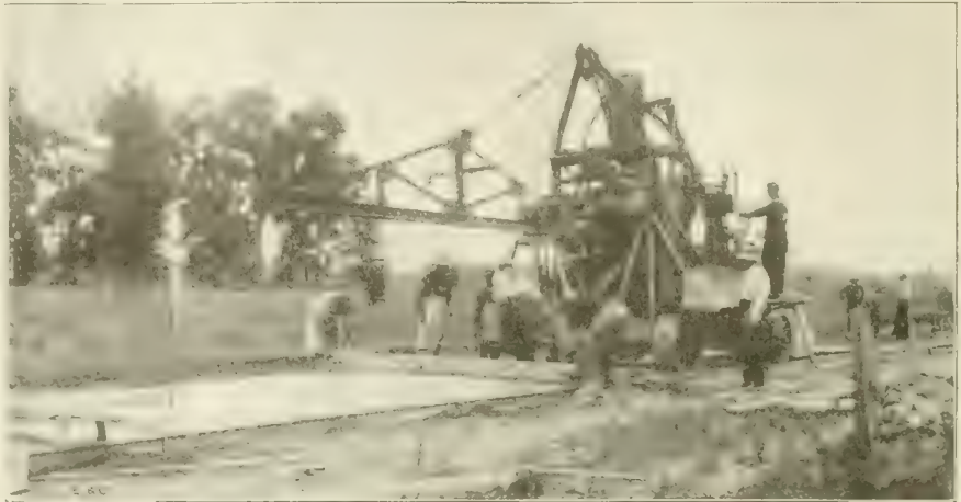
Fig. 2. Mixing and Placing Concrete. Note Steel Side Forms and Method of Finishing Surface.
