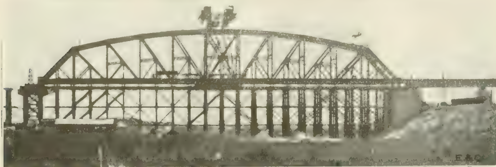
Fig. 5. View Showing Manner of Erecting South Truss Span of Lower Ganges Bridge— Note Falsework and Gantry Crane.
