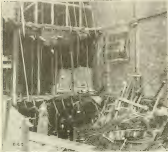
Fig. 2. View of Wrecked Portion of Theater and Arcade Building—Note Props for Floor and Stump of Column—See Fig. 1 for Location of Camera.
