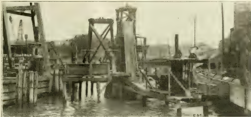
Fig. 10. View of Plant Used in Sinking Shaft, Mystic River Water Tunnel Extension.
