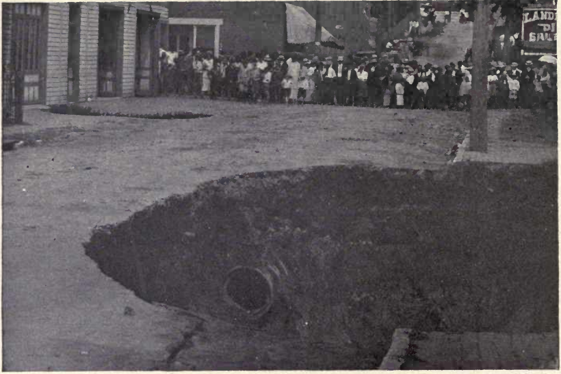
PLATE XLVIII, FIG. 1. — Street in Staunton, Va., showing sewer pipe whose break started the caving, and holes formed in pavement.
