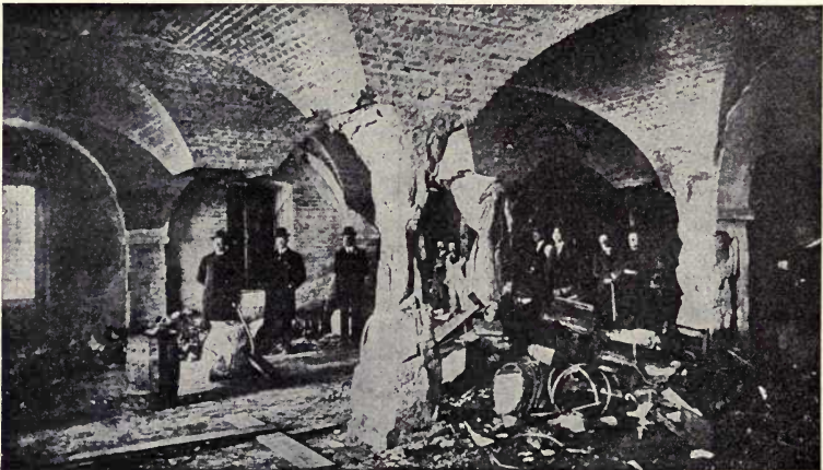
FIG. 195.—Effect of fire on granite columns, U. S. Public Storehouse, Baltimore, Md.
