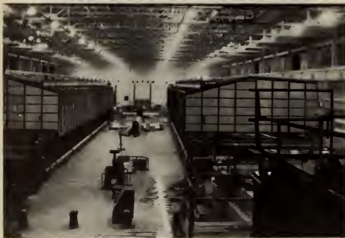
Fig. 10—General View of Paper Machine Room
