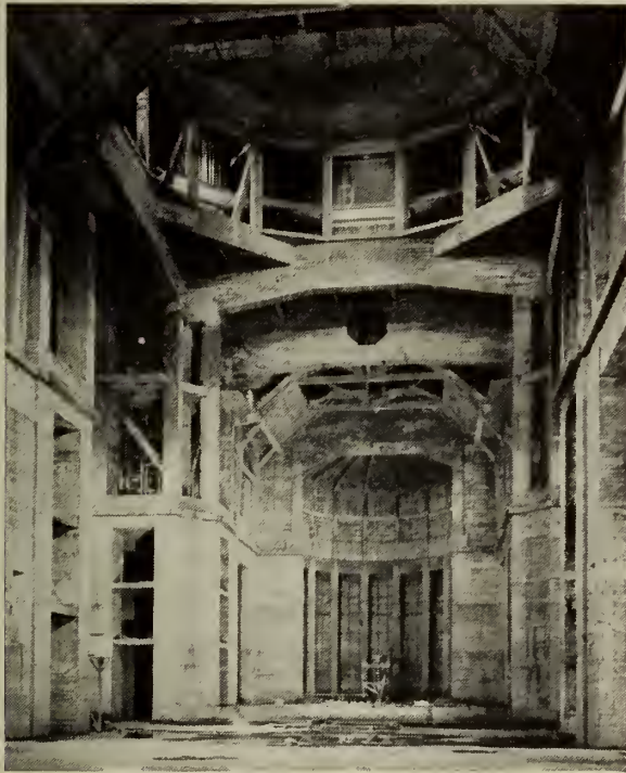
Fig. 8—Inside View of the Nave from the First Gallery Showing the Lower Facings of the Domes
