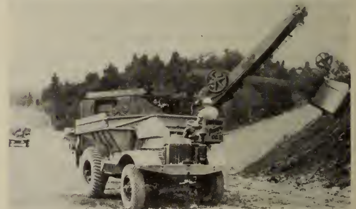
Fig. 8—Highway Work in New Brunswick, 1937. Heavy Earth Cutting Near Perth Using Dumptor and Gas Shovel
