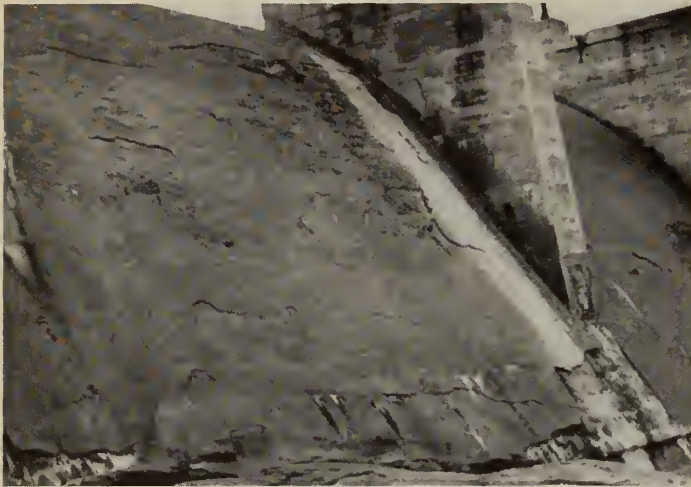
Fig. 4—Shows the present condition of gunite work which was done at La Gabelle in 1931. Dam built in 1924
