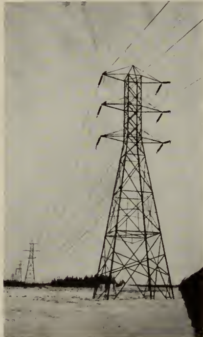
Fig. 4—Typical strain tower used on Port Alfred line
