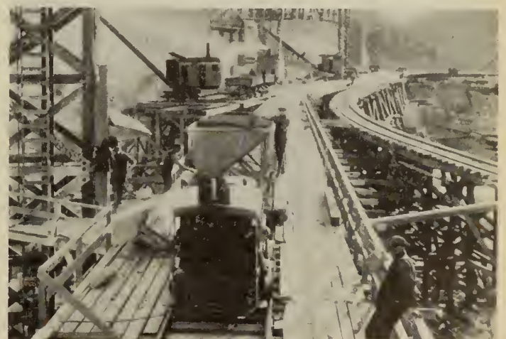
Fig. 2—La Gabelle development, 1922, Concreting Methods. Typical of this period concrete was transported from the mixing plant in special concrete cars or buggies and distributed by chutes from the concreting towers
