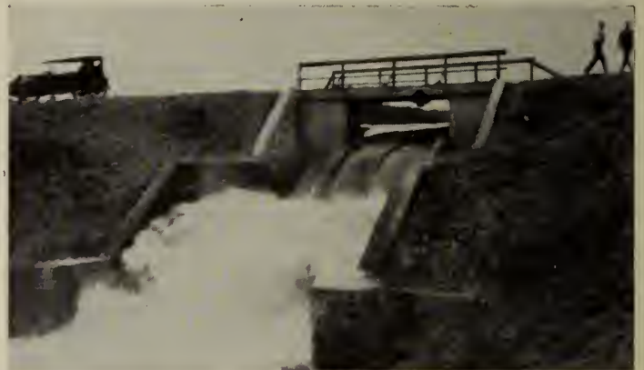
Fig. 2—Large concrete drop repaired and faced with glazed tile in 1924.
