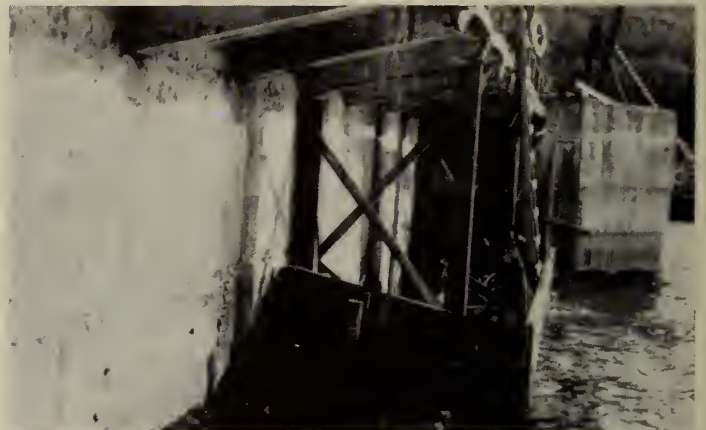
Fig. 5—Moving caisson being used on repairs to Gouin Dam shows the caisson in position against the upstream face of the dam. This dam was built in 1918
