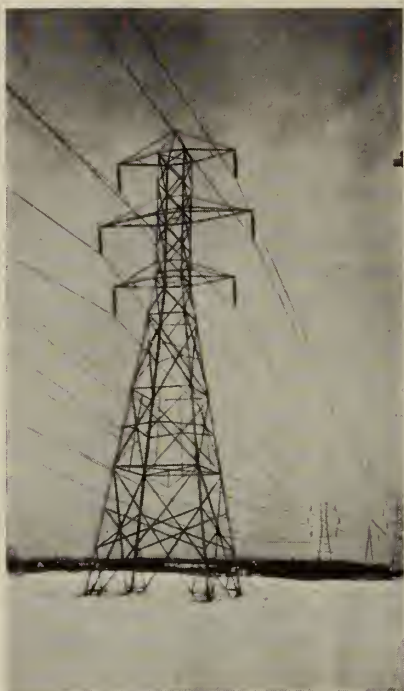
Fig. 2—Typical suspension tower used on Port Alfred line
