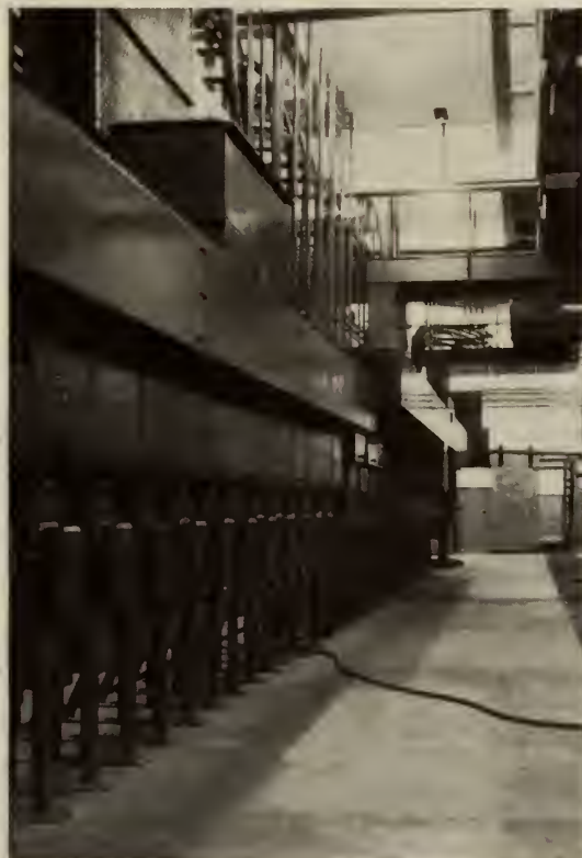
Fig. 8—Metal Clad Switchgear at Substation
