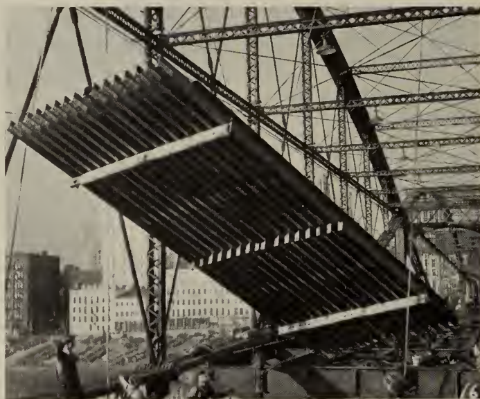
Fig. 6—A section of aluminum alloy floor being placed on the Smithfield Street Bridge in Pittsburgh, Pa.
