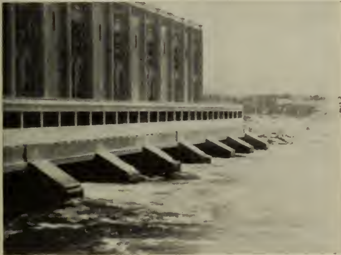
Fig. 1—Substructure of the powerhouse at Grand'Mère. The restoration work consisted of facing the heavy slab over the exits from the draft tubes and the tops of the piers supporting this slab together with considerable work which is concealed behind the barrier shown above the slab. It will be noted that this work is still apparently in perfect condition. The sides and noses of the piers were not repaired at that time and in fact it was not until last year that any repairs were made to this part of the structure. Built in 1918
