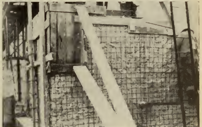
Fig. 3—Shows the placing of the wire mesh for gunite repairs to Almaville Dam in 1937
