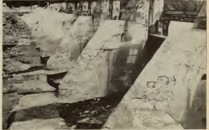
Fig. 2—Showing the deterioration that had taken place in unreinforced gunite placed on the piers of Almaville Dam in 1924. Dam built in 1910
