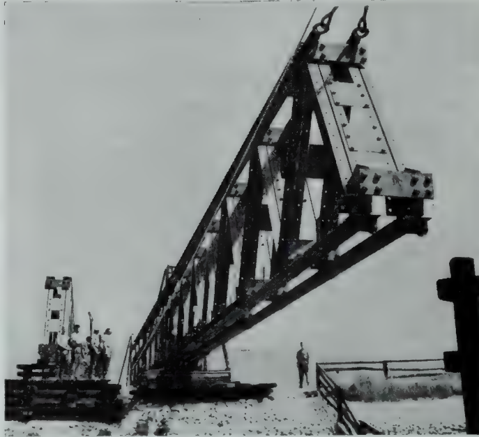
A new type bridge is under construction in Sussex. This is the first time the "derrick and preventor" method of launching has been carried out. Two double truss girders, each weighing 27 tons, and 140 ft. in length form the main part of the bridge. A derrick is erected to pull, by winch, the girders across the river. A cable and winch is secured to the opposite end to prevent the girder toppling when past point of balance. The first girder almost across. This is the most critical stage of the operation.
