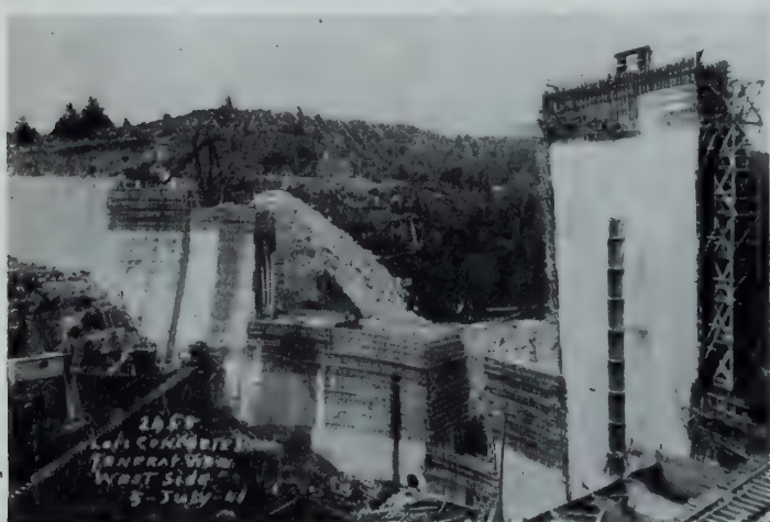
Fig. 3—General view of west side of dam showing entry gate section, culvert, and method of pouring successive sections.
