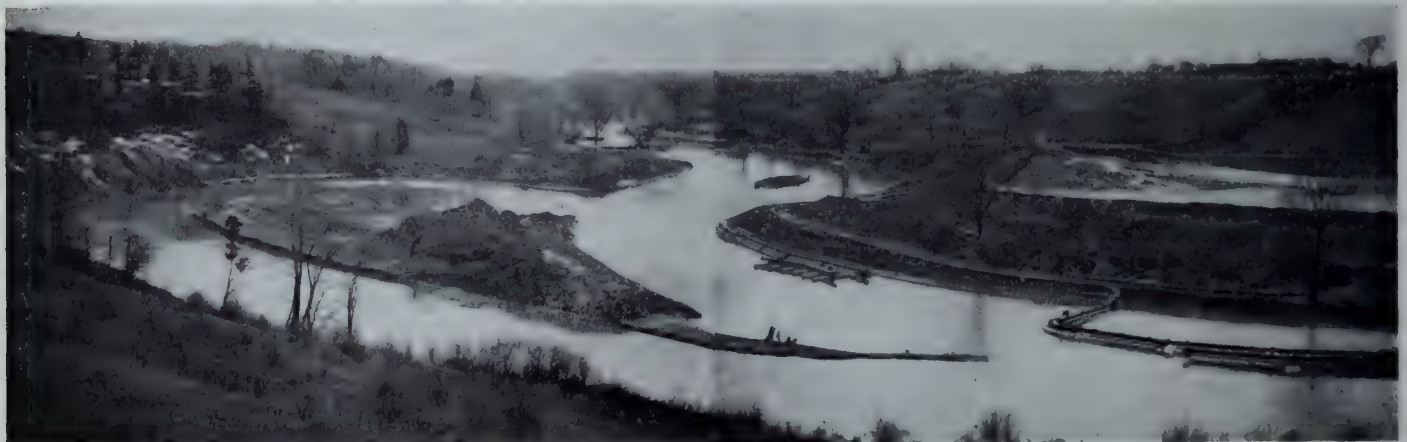
Fig. 10—Photographs of enlarged channel in Twelve Mile creek. Original channel at left, disposal area at right.
