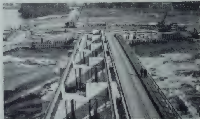
Construction of Dam No. 3 at Coteau (1943), showing first stage completed and opened, the second cofferdam unwatered, and the third section of the channel still flowing free.
