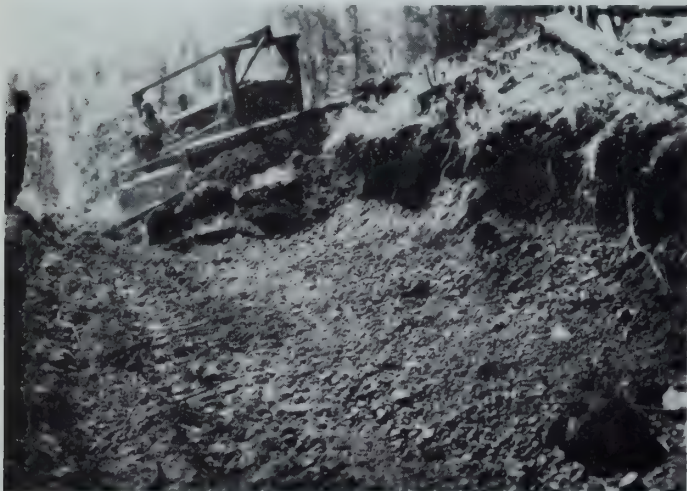
Rough grading sufficient to permit passage of truck traffic in weather not too wet.
