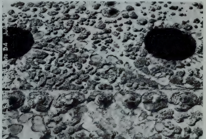
Close up view of rust tubercles. (Some of the tubercles have been scraped off.)
