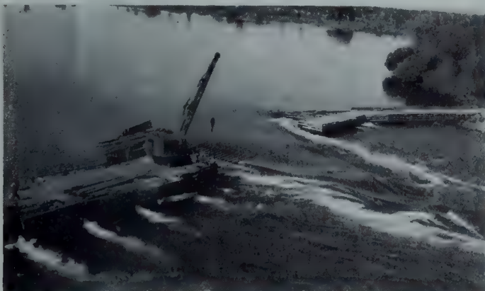
Closing the gap in the final stage of Coteau Dam No. 3 cofferdam.
