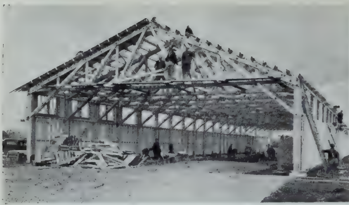
Fig. 16—51 ft. span triangular Pratt trusses which support a roof over a storage building for Fairchild Aircraft Ltd., near Montreal.
