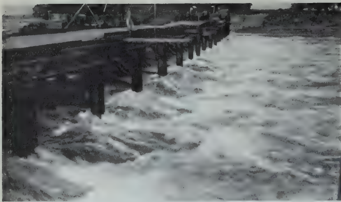
Steel cribs all placed across south channel at Ile Juillet with 20,000 cu. ft. per sec. flowing through open cribs prior to filling with rock.
