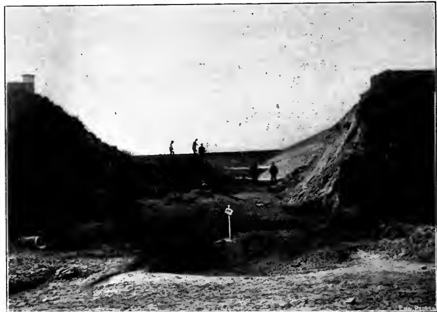
VIEW OF BREAK FROM OUTSIDE THE RESERVOIR.
