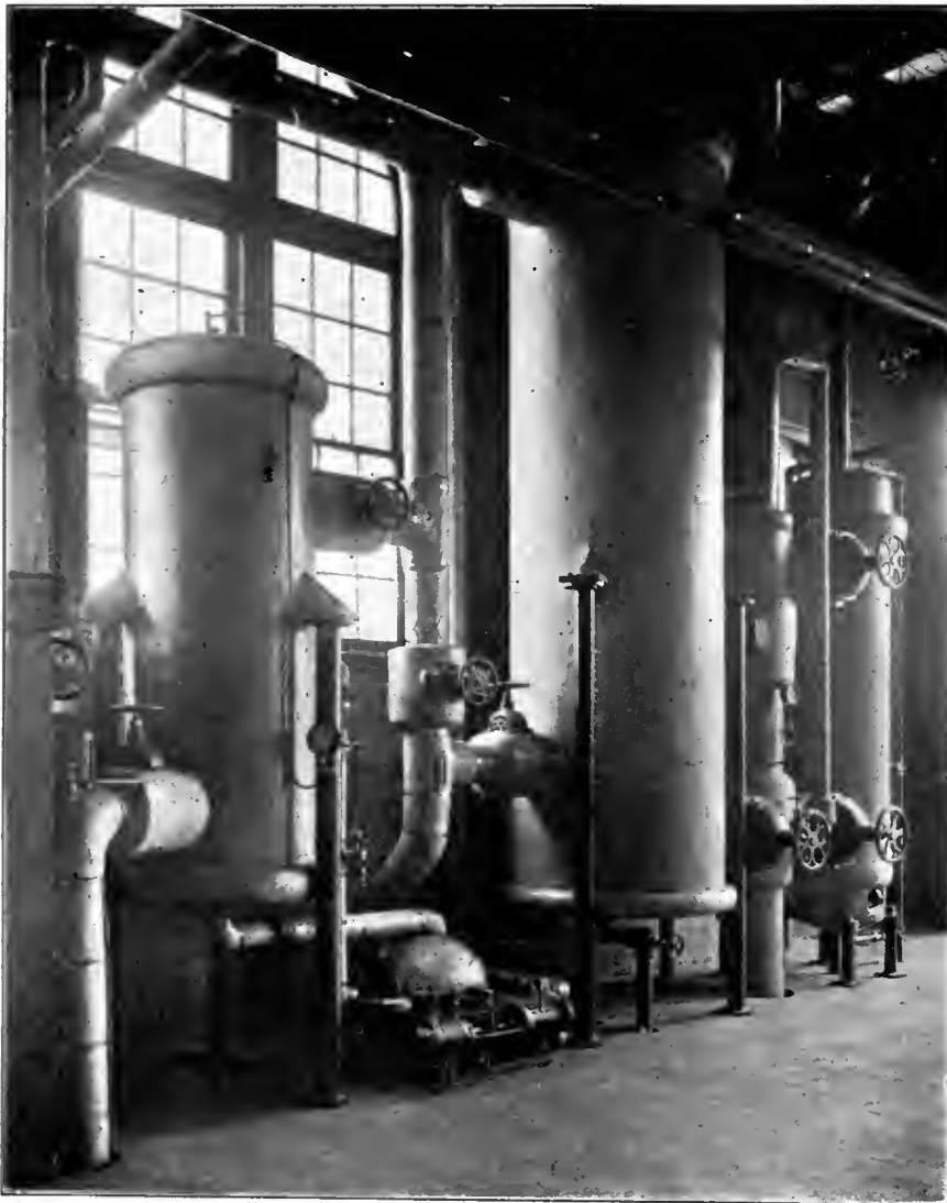
HEATERS IN POWERHOUSE FOR HOT-WATER HEATING SYSTEM.
