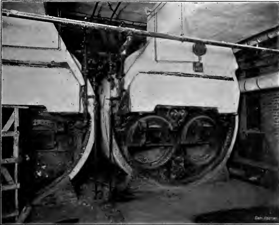
THE SCOTCH MARINE-TYPE BOILERS.
