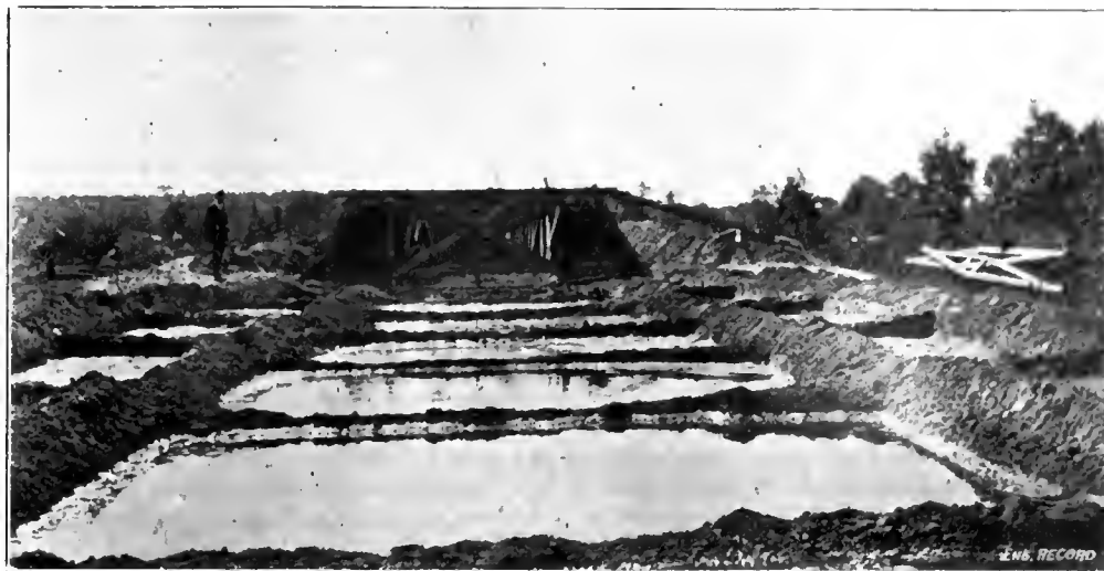
FLOODING FOUNDATION EMBANKMENTS FOR AQUEDUCT, FOR FINAL SETTLING, AFTER ROLLING IN THIN LAYERS.
