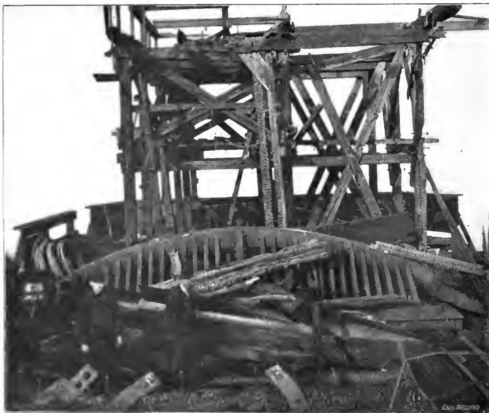
SADDLES AND WRECKED FALSEWORK ON NORTH SIDE OF TOWER.
