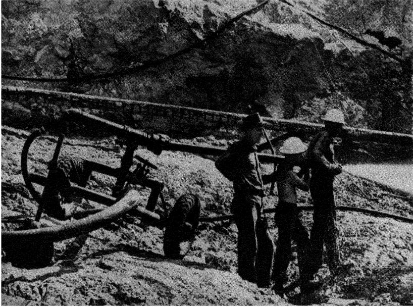
FIG. 30. Hydrauliclicking loose silt at Shasta Dam preparatory to drilling. A 3-inch manifold hose is shown in foreground; the smaller hose is a 1-inch air hose. (Photograph from U.S. Bureau of Reclamation.)
