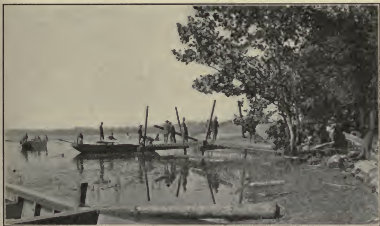
FIG. 10.—Constructing bridge by successive pontoons. Two trestles are placed, and the first ponton with saddle in center is in position.
