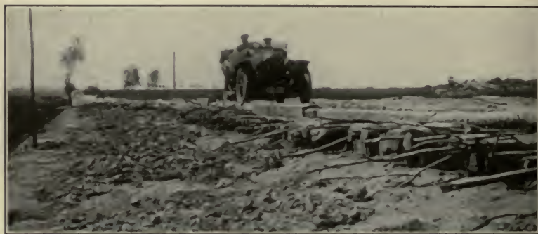
FIG. 28.—Road improved for military use by paving of logs and brush. Constructed by the Germans in Russia.
