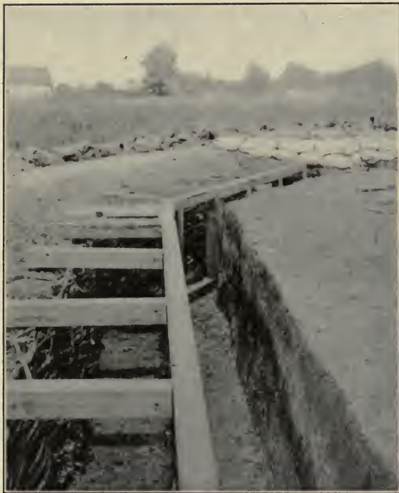
FIG. 39.—Shelter under parapet in construction. Timber frame and covering of sand-bags on plank.
