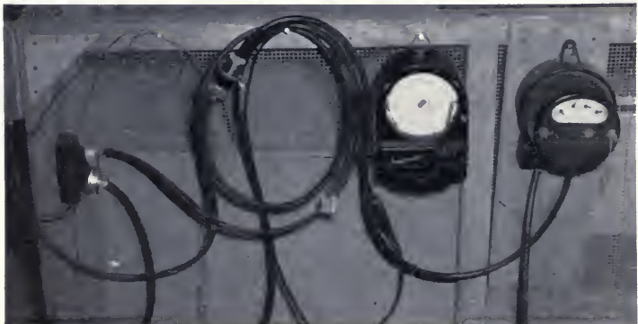
Tempscribe on-off recorder and watt-hour meter used in all tests. (Fig. 12)
