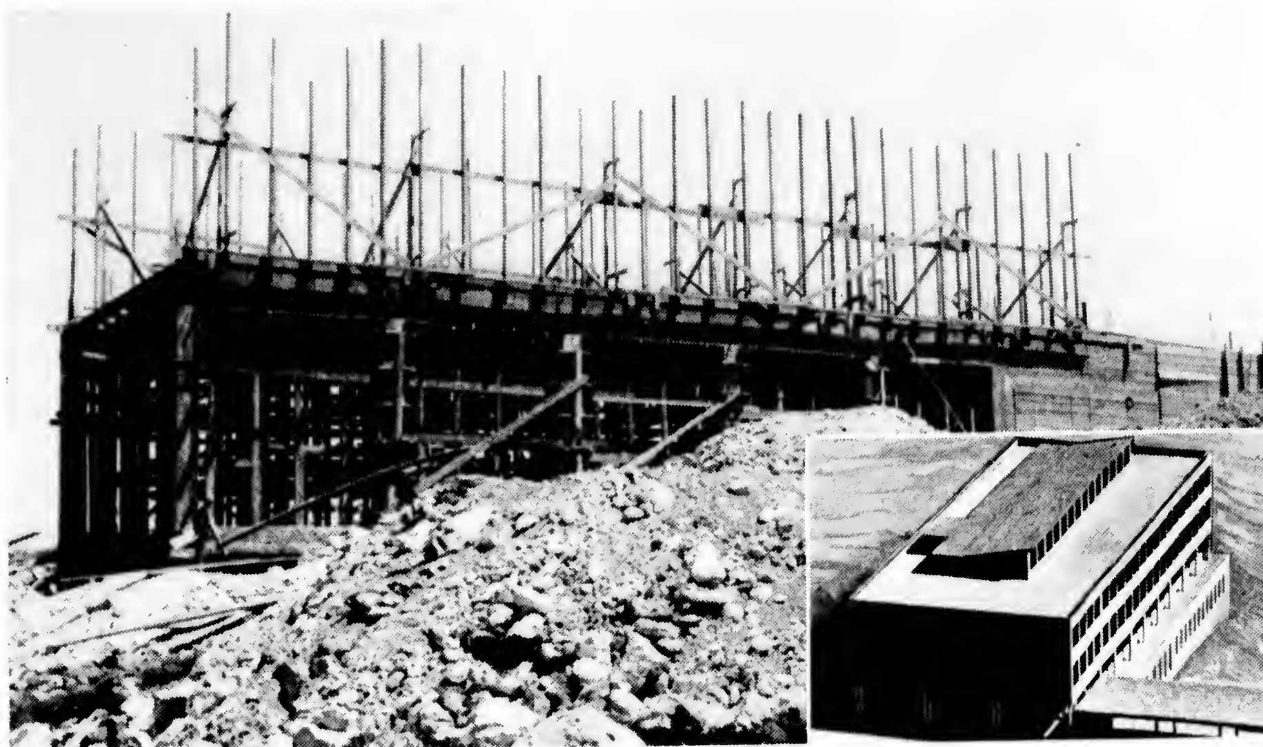
Construction of the campus at Givat Ram continues at a feverish pace, ahead of schedule. Inset shows architect's drawing of how the Abraham Mazer Memorial Building, which will house the Institute of Jewish Studies, is to look on completion. It is expected that this structure will be completed by the end of 1956.
