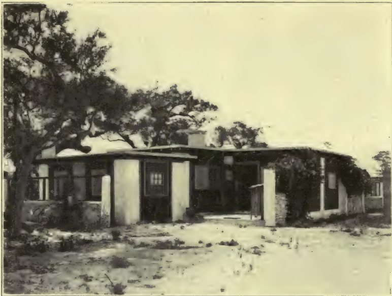
A UNIT OR PUEBLO HOUSE IN PROCESS OF CONSTRUCTION. CONCRETE ROOF AND CONCRETE FLOORS. THIS HOUSE CONSISTS OF THREE UNITS JOINED TOGETHER ON A TRIANGULAR LOT. VIEW FROM SOUTHWEST. (PHOTO BY KAUFMAN, MIAMI, FLA.)
