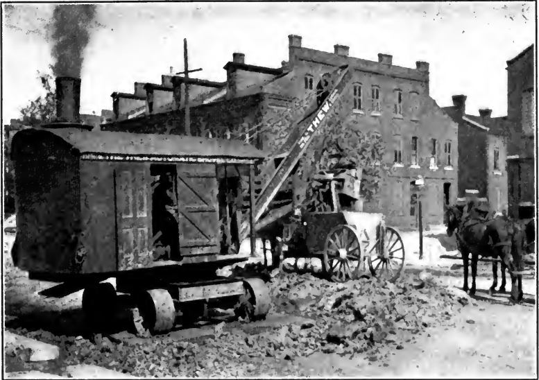
FIG. 137.—Steam shovel removing old street surface. (Courtesy of The Automatic Shovel Co.)
