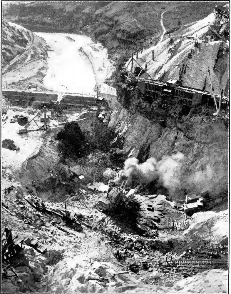
FIG. 162.—Excavation of foundation for Arrowrock Dam. (Courtesy of U. S. Reclamation Service.)
