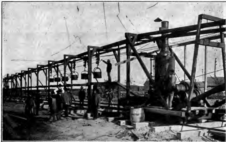
FIG. 70.—“Carson-Trainor” trench excavator on sewer trench construction. (Courtesy of Carson Trench Machine Co.)
