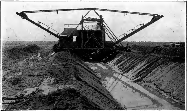
FIG. 60.—Austin templet excavator with narrow bottom frame. (Courtesy of F. C. Austin Co.)
