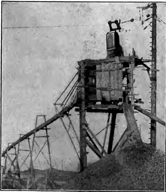
FIG. 82.—Cableway excavator operating at gravel pit. (Courtesy of Indianapolis Cable Excavator Co.)
