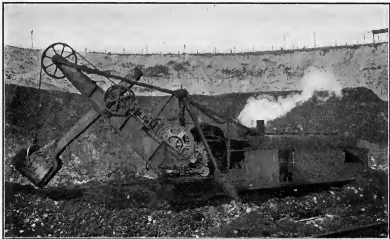
FIG. 200.—Atlantic type steam shovel excavating iron ore. (Courtesy of The Bucyrus Co.)
