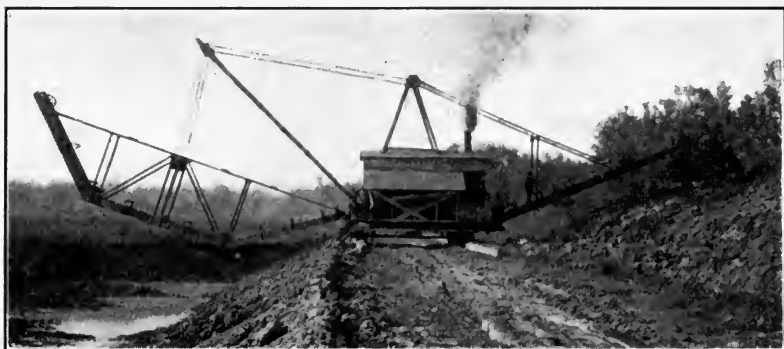
FIG. 169.—Austin templet machine constructing a levee. (Courtesy of F. C. Austin Co.)
