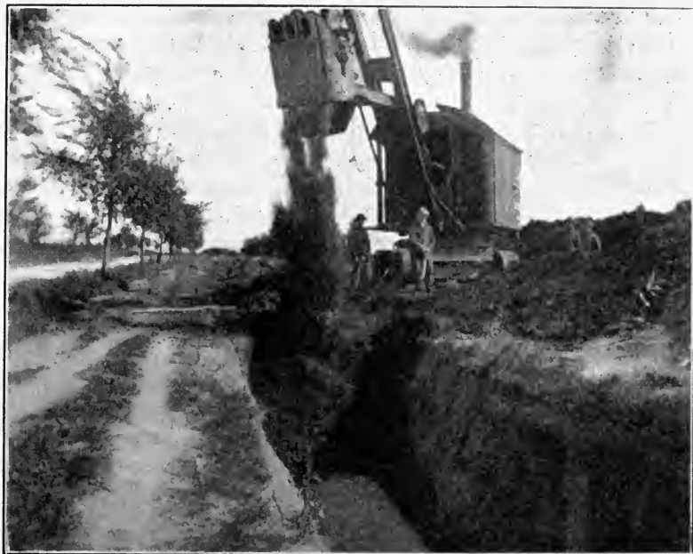
FIG. 180.—Revolving steam shovel backfilling large trench. (Courtesy of City Engineer, Minneapolis, Minn.)
