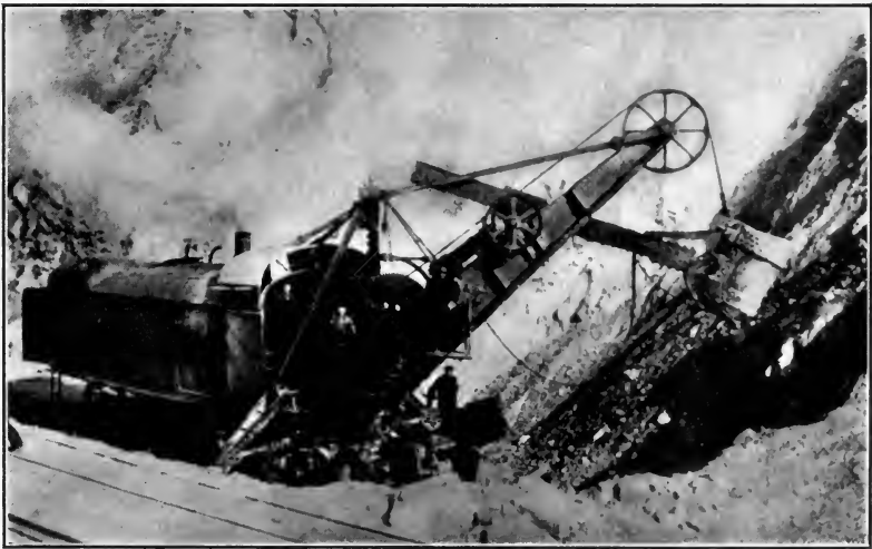
FIG. 161.—Atlantic steam shovel excavating foundation of Arrowrock Dam. (Courtesy of the Bucyrus Co.)
