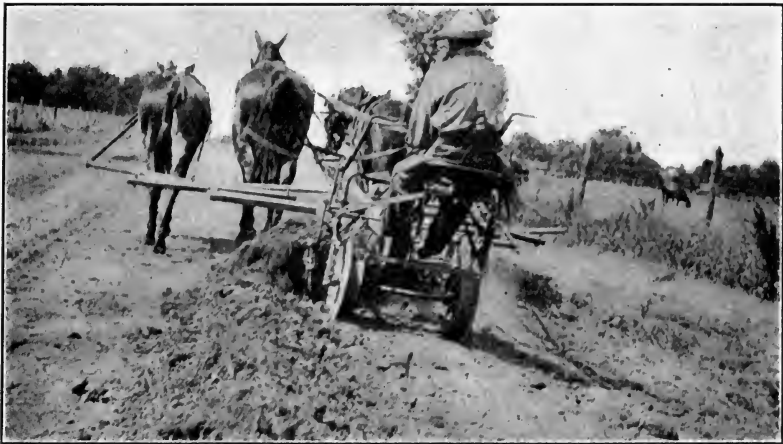
FIG. 131.—Two-wheel grader shaping up a road. (Courtesy of the Baker Mfg. Co.)
