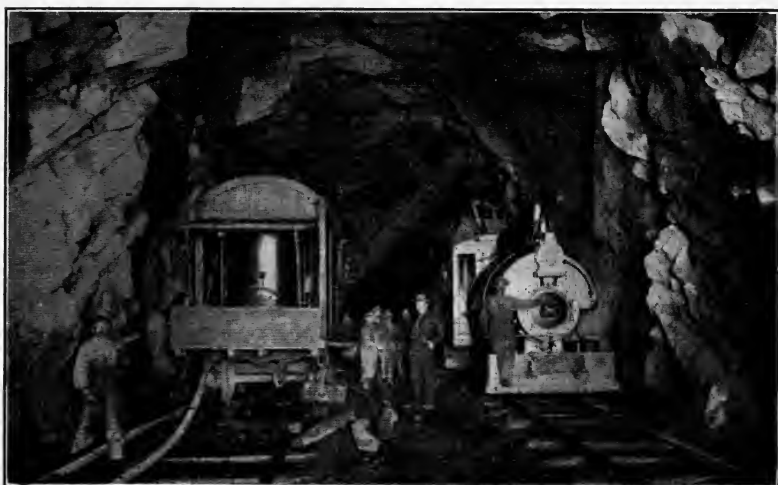
FIG. 208.—Power shovel operating in Bergen Hills tunnels. (Courtesy of Marion Steam Shovel Co.)
