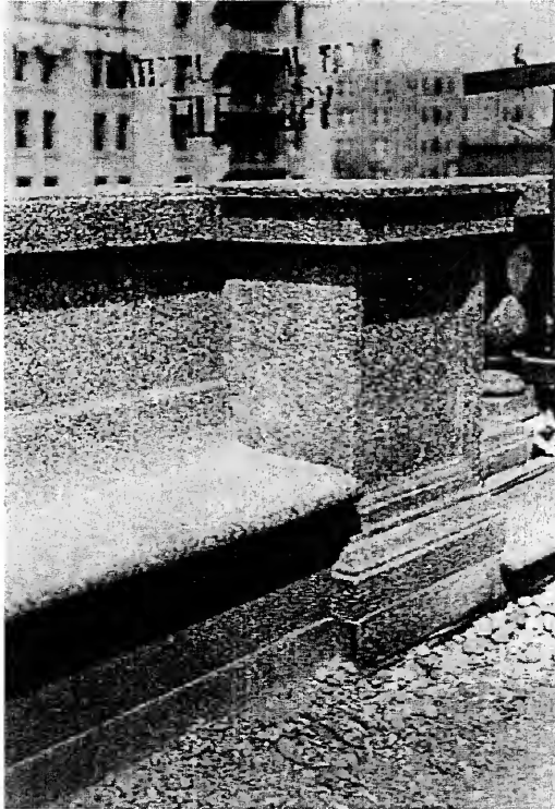
Figure 23: Main 16 th Street Entrance Overlook Area, Molded Benches, n.d (c. 1918-19) Rock Creek Park, Cultural Resource Management Archives
