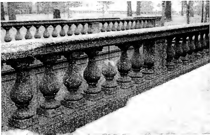
Figure 53: Losses from Cracked Balusters, West Balustrade above South Steps, Main 16 th Street Entrance
