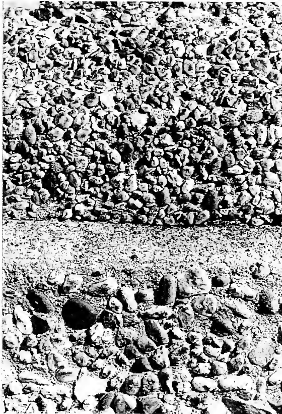
Figure 59: Thin Black Crust on Exposed Aggregate
