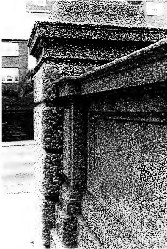
Figure 64: Current Condition of Concrete Work at Meridian Hill Park
