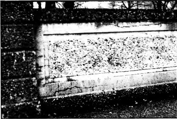
Figure 54: Location of Efflorescence on West Wall Panel
