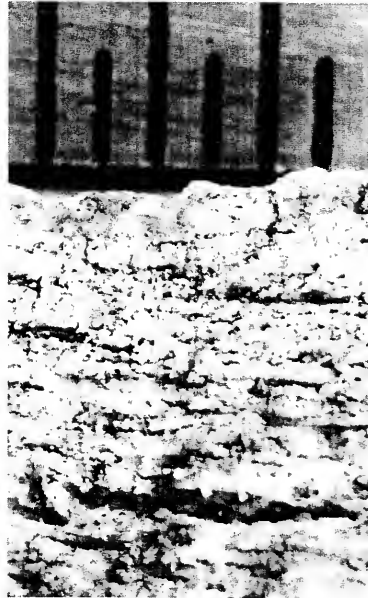
Multiple Layers of calcreous efflorescence at joints
