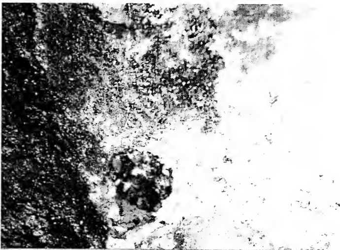
Corrosion Products on Interior Surface
