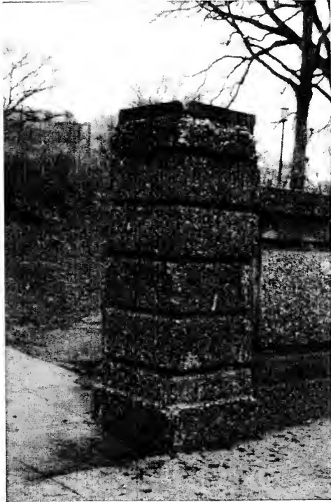
Figure 44: Spalling on South Post of Northwest Entrance
