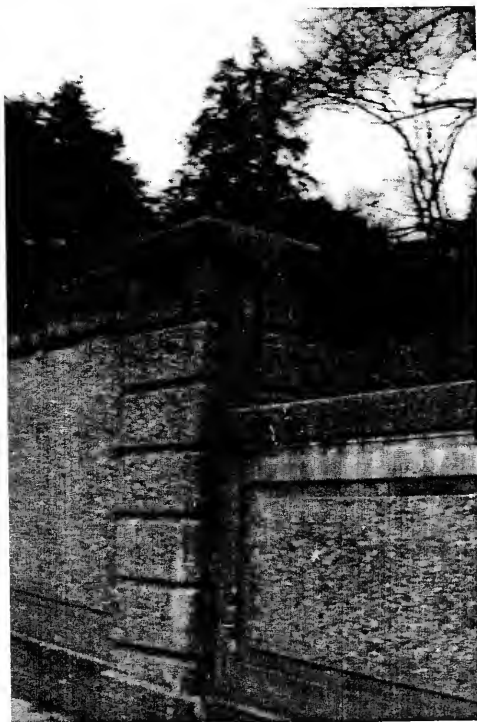
Figure 18: Missing Console from West Wall
