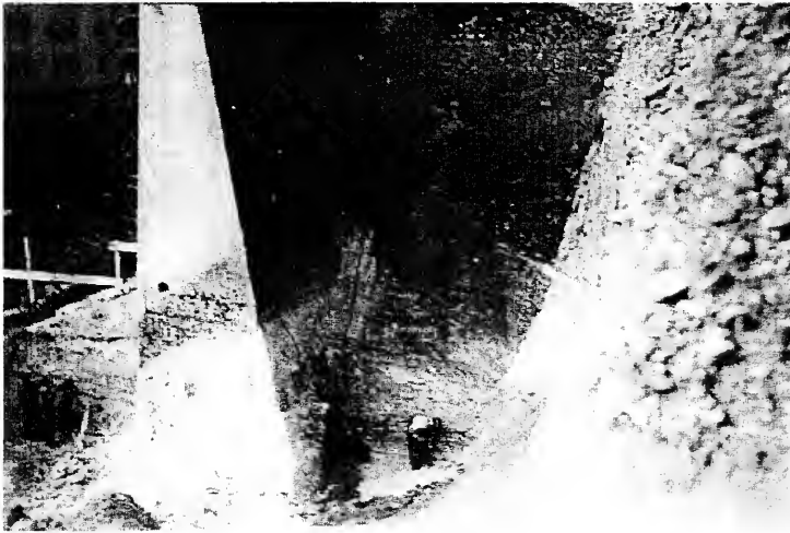
Figure 25: Upper 16 th Street Retaining Wall Footing, c. 1929 Rock Creek Park, Cultural Resource Management Archives
