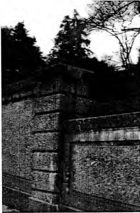
Figure 50: Missing Console from West Wall
