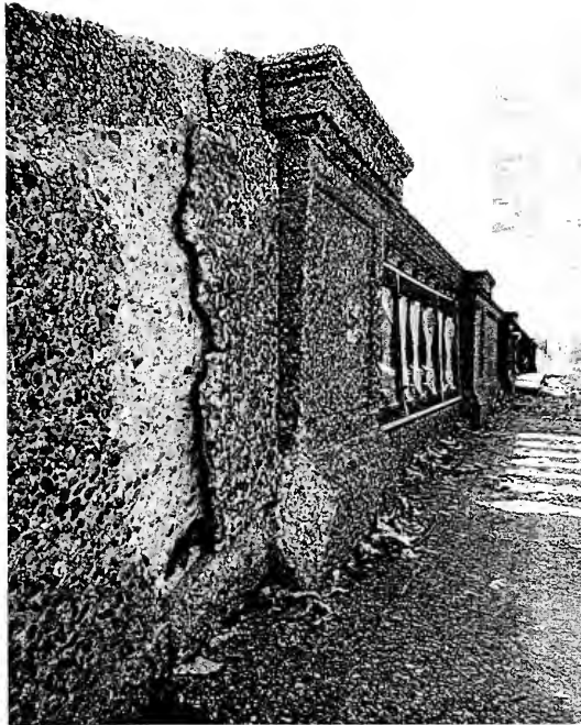
Figure 33: Spalling and Delamination on Upper Retaining Wall Balustrade, 1964 Note: Mesh cover over balustrade openings NPS MARS Collection
