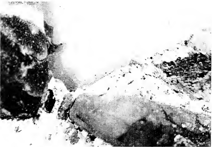
Figure 36: Non-eroded surface, Interior of Main 16 th Street Entrance
