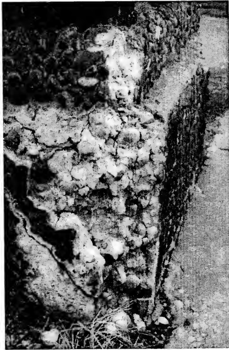
Figure 42: Spalling and Delamination, Base of South Post of Northeast Entrance
