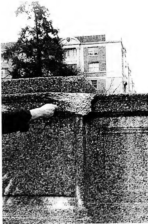
Figure 46: Spalling at edge of coping on upper south post of Lower 16 th Street Entrance
