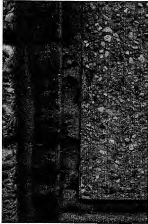
Figure 57: Black Gypsum Crusts on Wall Panel Note: Absence of crust at joint where water flows
