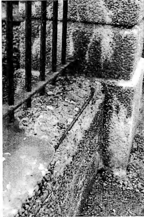
Figure 45: Spalling on top of low North Wall and failure of drip edge
