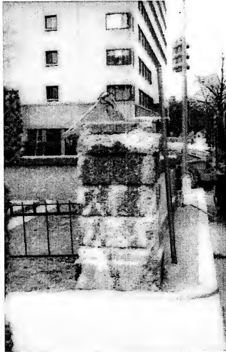
Figure 41: Spalling and Delamination, North Post of Northeast Entrance
