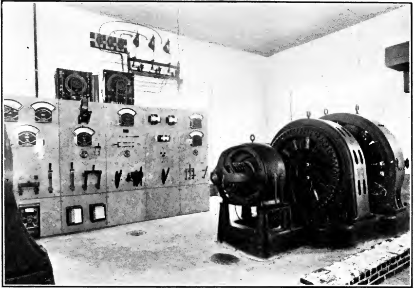
FIG. 1.—MOTOR GENERATOR SET AND SWITCHBOARD.
