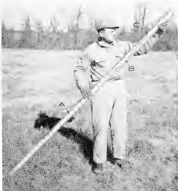
FIG. 538.—Method of assembly to prevent strain on cap wires. A, cartridge of explosives; B, cap wires; C, half hitch loop to take strain.
