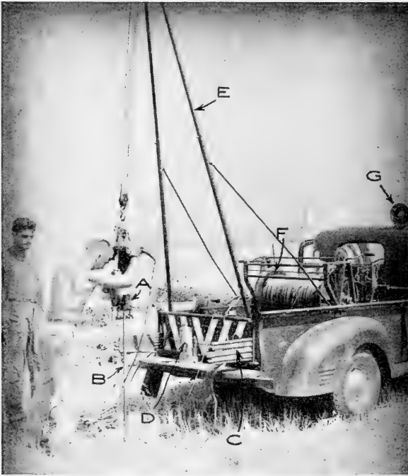
FIG. 316.—Driving long electrodes with power-driven hammer. A, gasoline hammer; B, 6-foot, tapered steel electrode; C, spare electrodes; D, hydraulic jack for withdrawing electrode; E, folding "A" frame for supporting hammer; F, reel carrying insulated wire; G, loud speaker for short wave radio communication. (Courtesy of Union Oil Company of California.)
