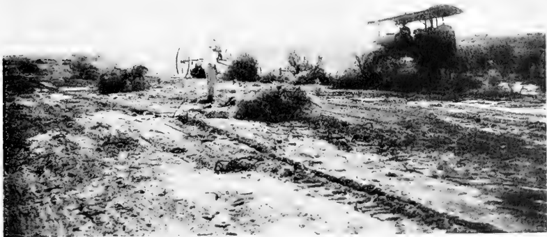
FIG. 163.—Greasewood and catchlaw offer no obstacle to the giant grading machines employed on the San Carlos project.
