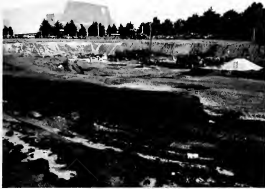
The construction site is located on what was formerly the faculty and student parking lot. Students now find alternative parking at Good Shepherd.
