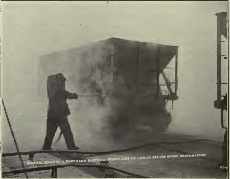
Fig. 11.—Hood used by men sand-blasting steel ore cars. Duluth, Missabe and Northern Railway.
