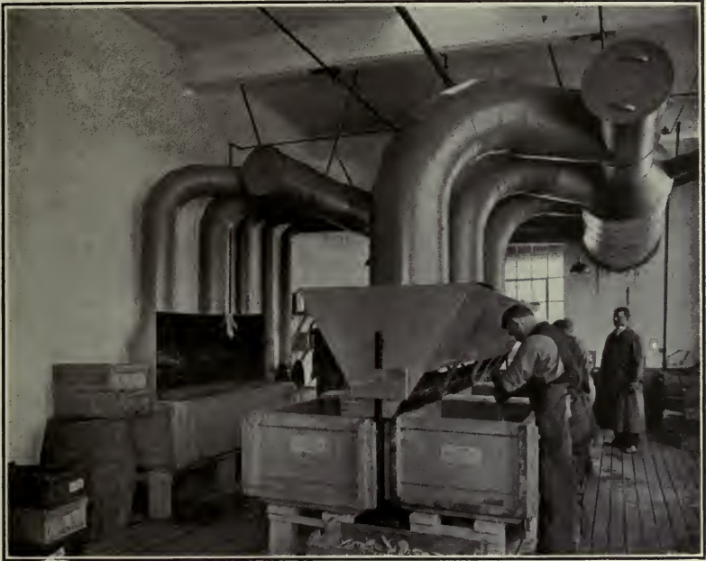
Fig. 33.—Ventilating System for Removing Acid Fumes. The suction opening is below the operator's breathing line, and no fumes reach his face. American Museum of Safety.
