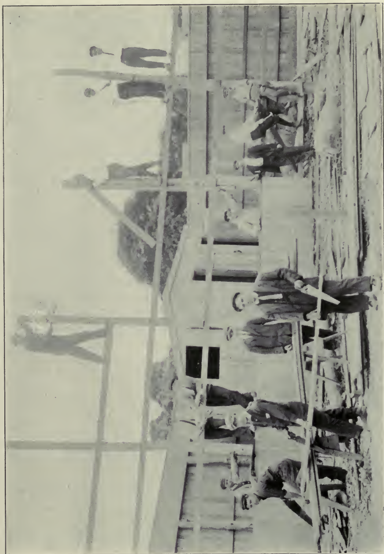
FIG. 7. NEW BEDFORD, MASS., INDUSTRIAL SCHOOL FOR BOYS. FENCE ENCLOSING GENERAL ATHLETIC FIELD UNDER CONSTRUCTION BY INDUSTRIAL SCHOOL PUPILS.
